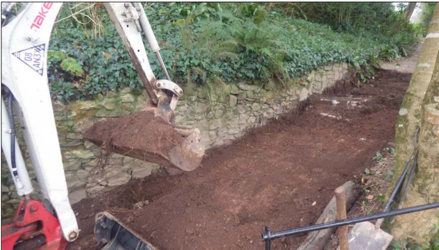
Plate 2: Working view during removal of Dunster Steps 1 (Lower Steps). View to south
