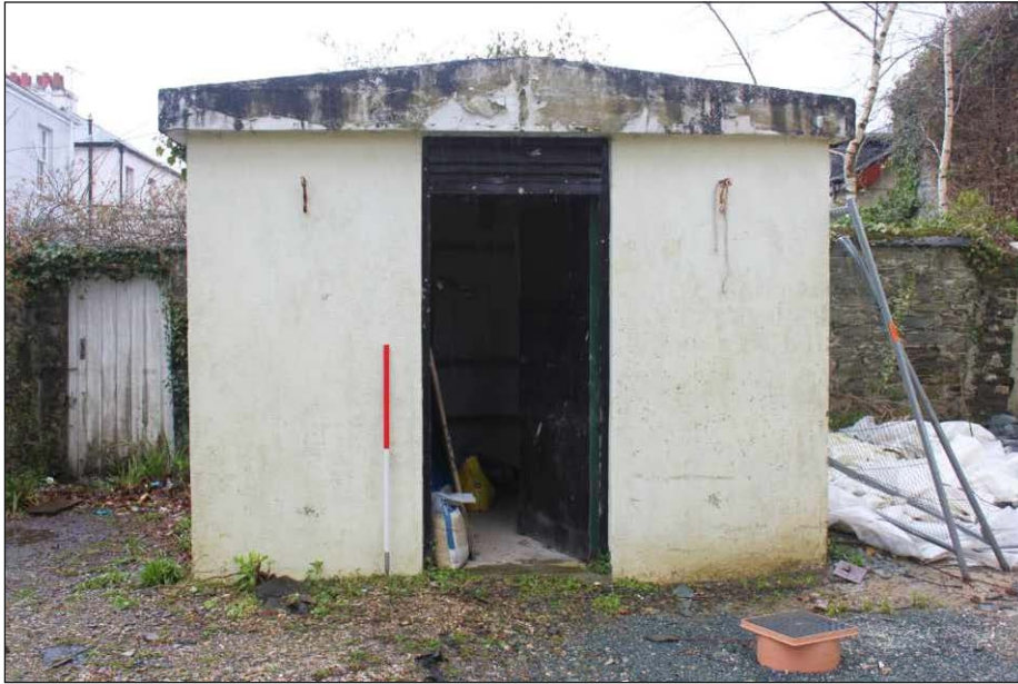
Plate 5: The northeast elevation showing the doorway with slatted vent above, looking southwest (1m scale)
