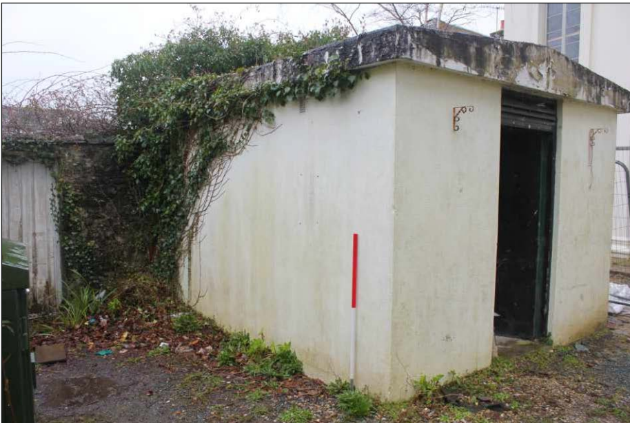
Plate 2: The outbuilding showing the vents in the southeast elevation, looking northwest (1m scale)
