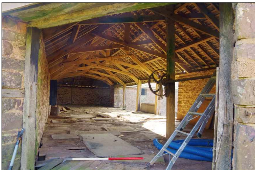
Plate 6: General view of the first floor of the north range, showing the drive shaft and end pulley wheel on the right, looking east (1m scale)
