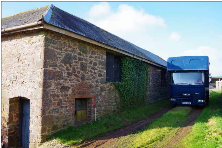
Plate 2: General view of east end of north elevation of the north range, looking southwest (1m scale)
