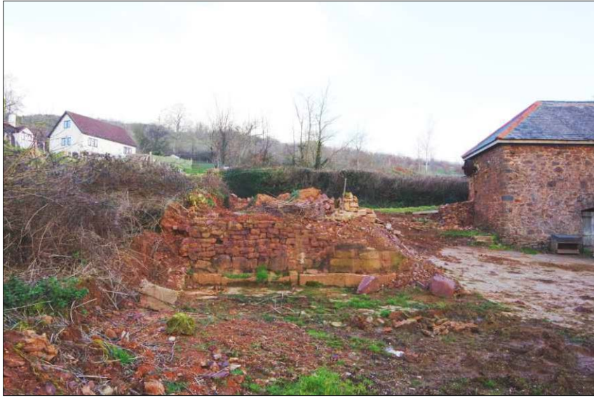
Plate 16: General view of former threshing barn, showing remaining south wall, looking north
