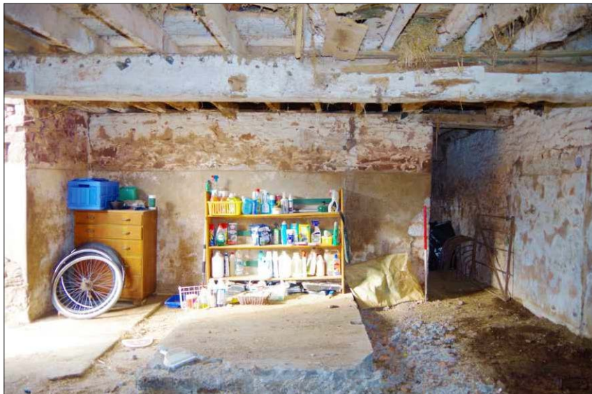
Plate 5: General view of the central livestock area in the north range, looking west (1m scale)
