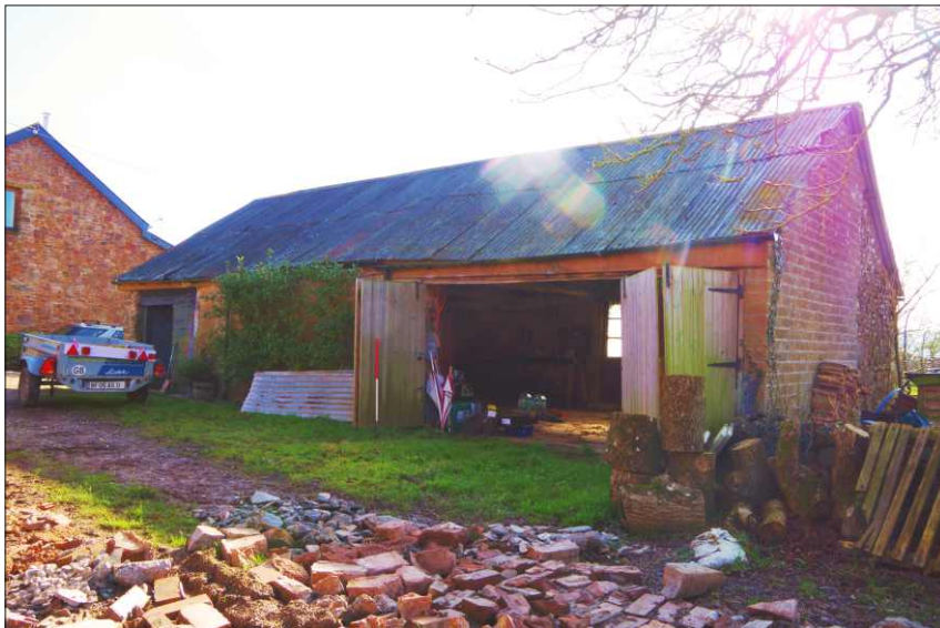
Plate 17: General view of the north and west elevations of the garage/store, looking southeast (1m scale)
