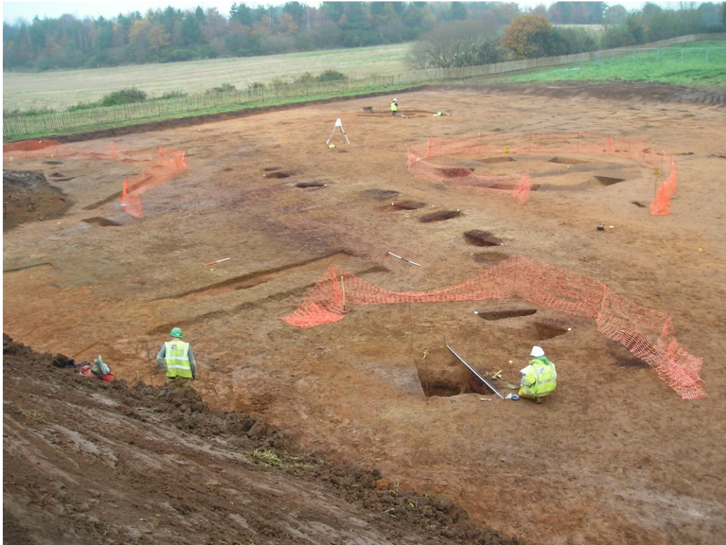
Fig. 10: Area A, work in progress, looking north, with ring ditch F1013 middle right [AC archaeology]
