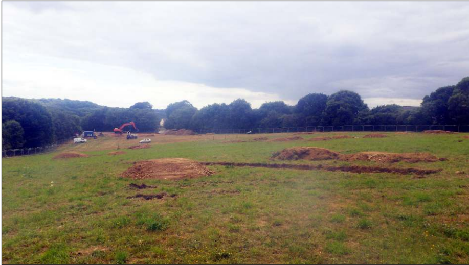
Plate 1: General view of the site with Trench 2 in the foreground, looking southwest
