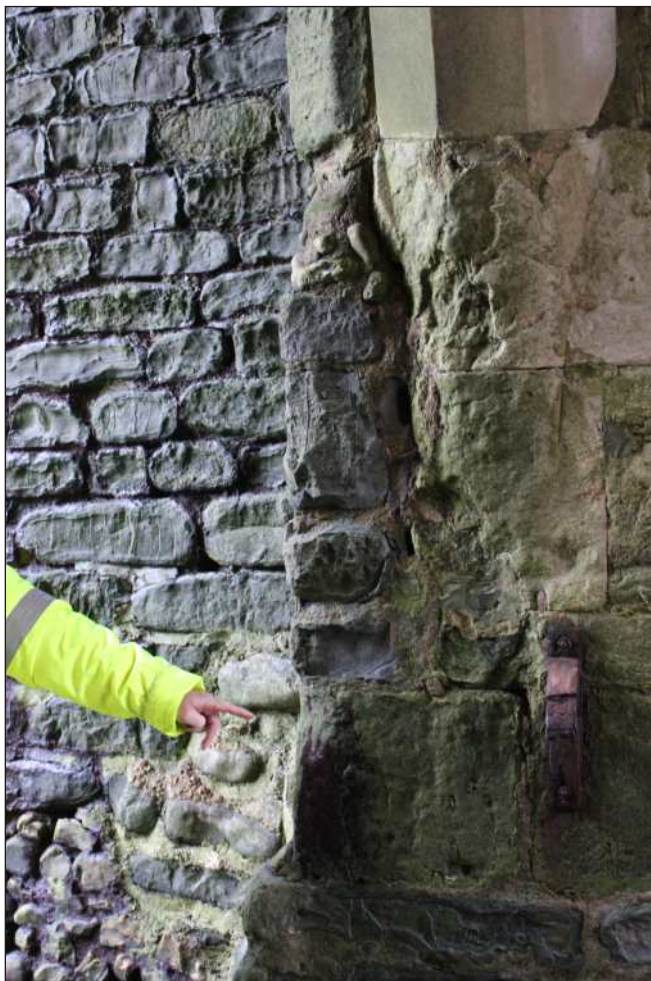
Plate 10: Eroded chamfer stop on the south end of the bridge on the east side
