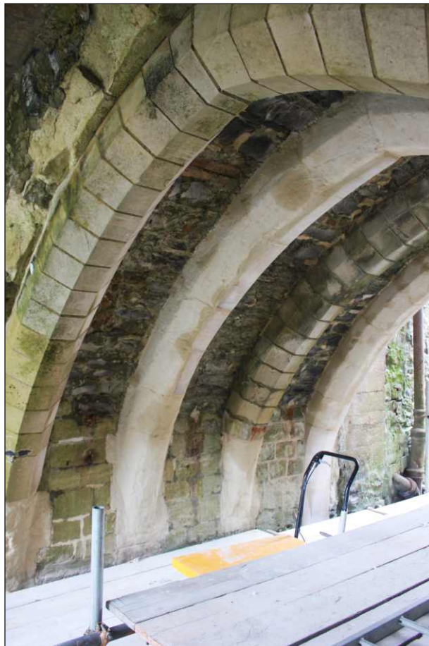
Appendix Plate 14: Rib 3, west side of south face following completion of repairs, viewed from the south
