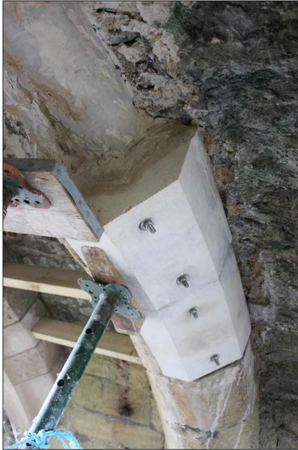
Appendix Plate 5: Rib 3 showing replacement voussoirs with pins, viewed from the north
