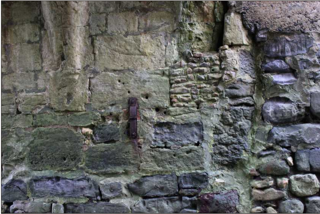
Plate 11: Repairs at the base of Rib 1 on the west side of the bridge
