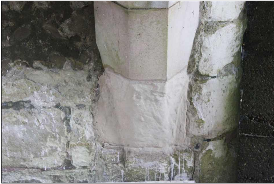
Appendix Plate 15: Rib 4, east side following application of shelter coat, viewed from the southwest
