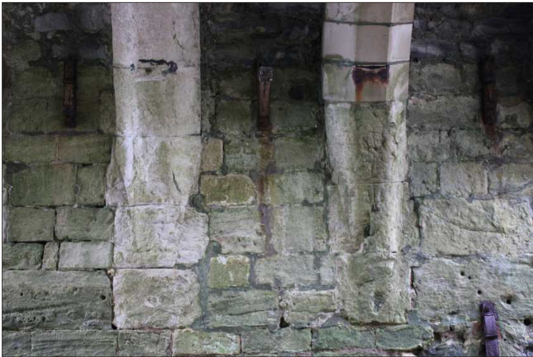
Plate 12: Dressed masonry between ribs 2 and 3 on the west side of the bridge
