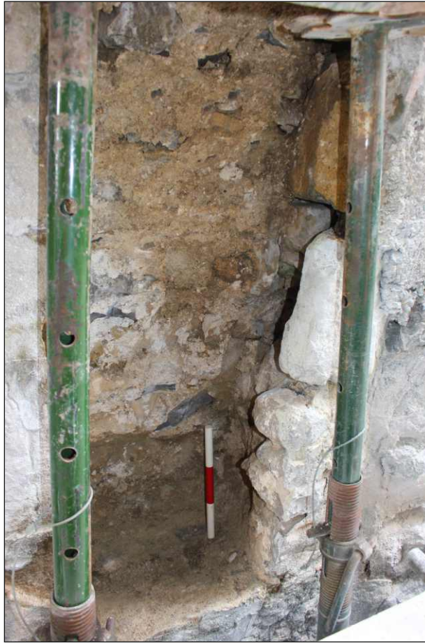
Appendix Plate 19: Rib 1 following removal of stones 1W:3 and 1W:4 and repair 125 showing the inside of the ring arch and abutting lias masonry 104, viewed from the east. (0.3m scale)
