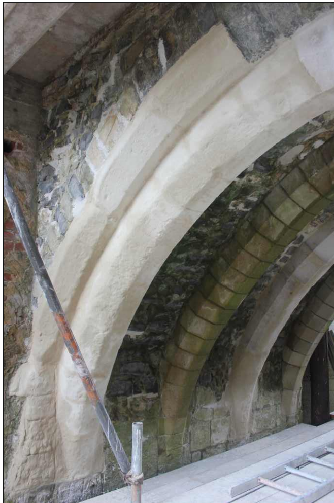
Appendix Plate 8: Rib 1, east side of north face following completion of repairs, viewed from the northwest
