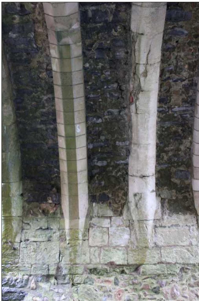
Plate 8: Roughly dressed blue lias stone between ribs 2 and 3 on the east side of the bridge
