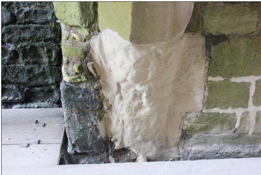
Appendix Plate 16: Rib 4, west side following application of shelter coat, viewed from the northeast
