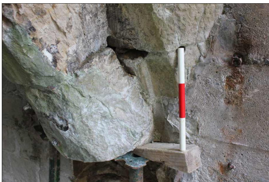
Appendix Plate 18: Rib 1 showing stones 1W:5 and 1W:6 with the projecting ring arch to the right (behind the 0.30m scale), viewed from the north
