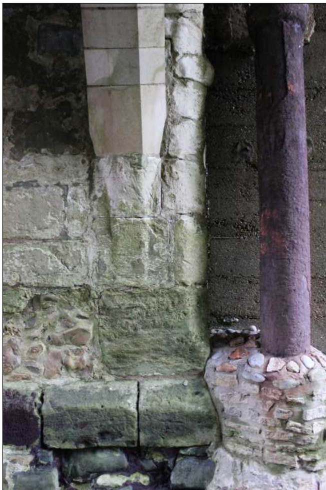
Plate 6: The run-out stop forming the base of chamfer on the south end of the bridge on the east side
