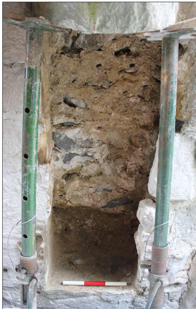
Appendix Plate 2: Rib 1 following removal of damaged lower voussoirs, viewed from the northeast. (0.30m scale)
