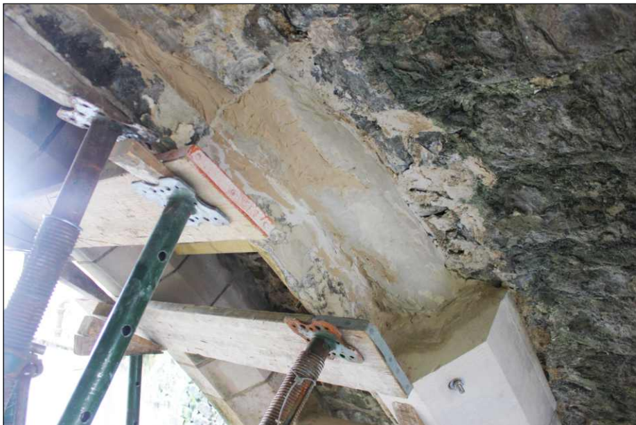
Appendix Plate 4: Rib 3 showing voids in masonry filled with mortar, viewed from the north
