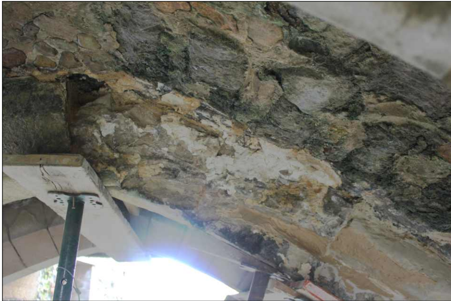
Appendix Plate 3: Rib 3 following removal of some of the damaged voussoirs, viewed from the northwest
