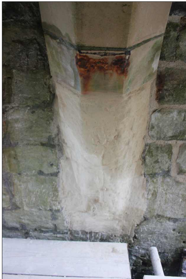
Appendix Plate 12: Rib 2, west side following application of shelter coat, viewed from the northeast
