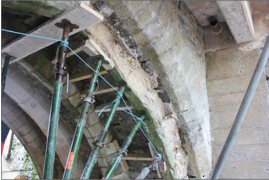
Appendix Plate 1: Rib 1 following removal of damaged elements of voussoirs, viewed from the north
