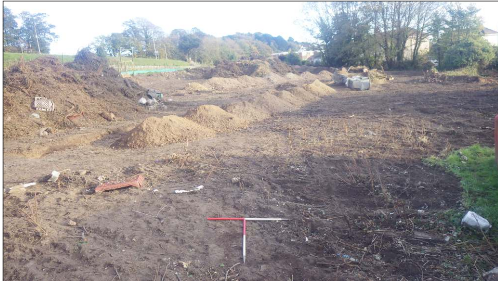
Plate 11: General view of the site in the area of Trench 5, looking northwest (1m and 1m scales)
