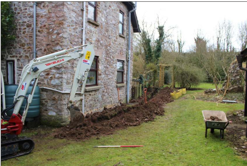
Plate 5: General view of excavations along north side of the Manor House. View to west (scale 1m)
