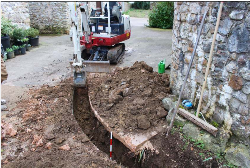
Plate 2: Working view of excavations through top of moat F1011 deposits. View to south (scale 0.5m)
