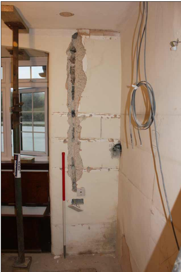
Plate 4: The interior face of the east elevation of the mill house prior to removal of finishes, looking northeast (1m scale)
