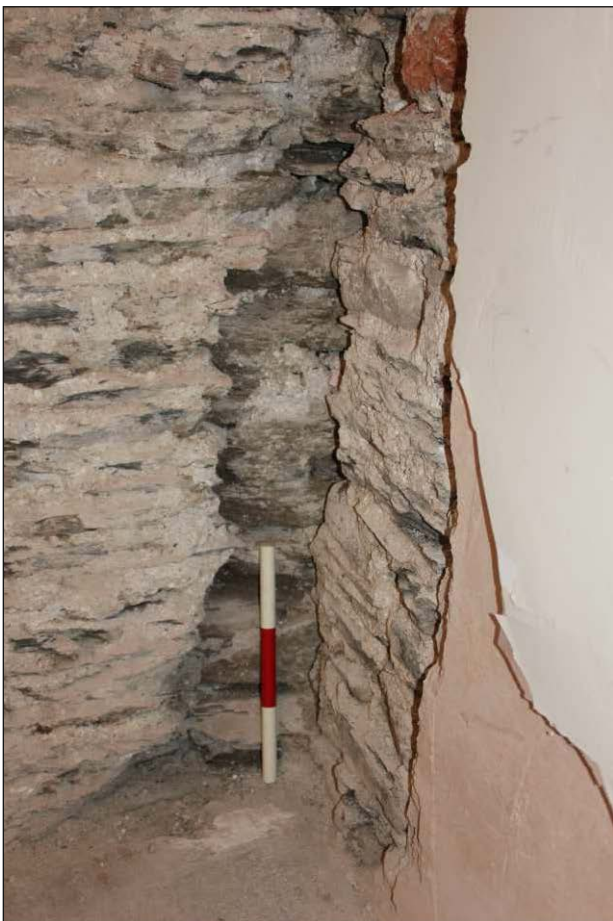
Plate 6: The primary curving masonry of the tide mill exposed within the mill house, looking east (0.30m scale)
