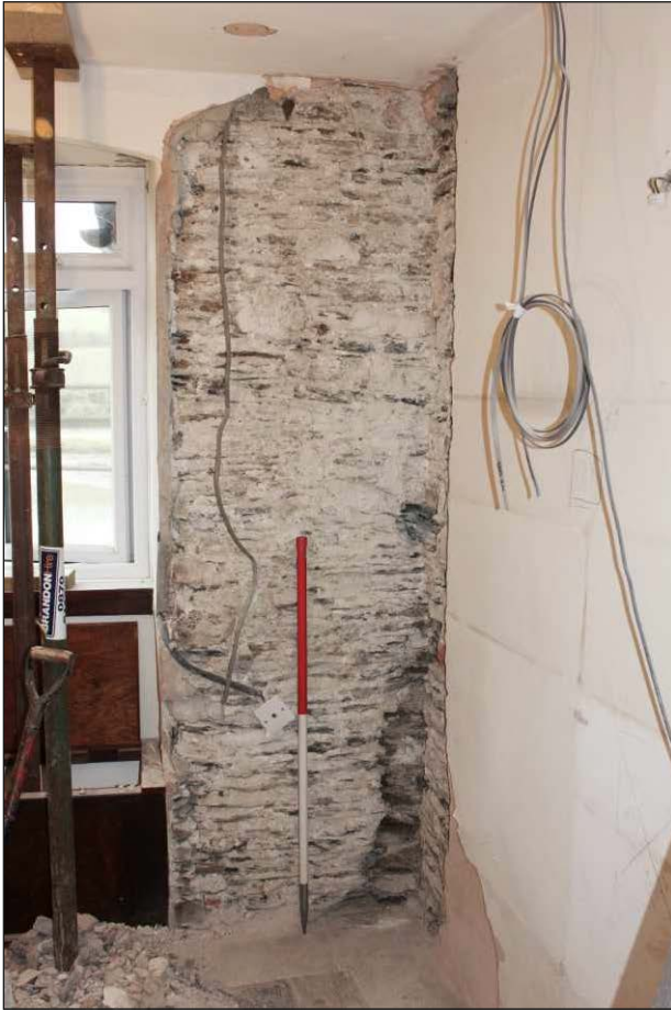
Plate 7: The masonry of the mill house following removal of plaster, looking northeast (1m scale)
