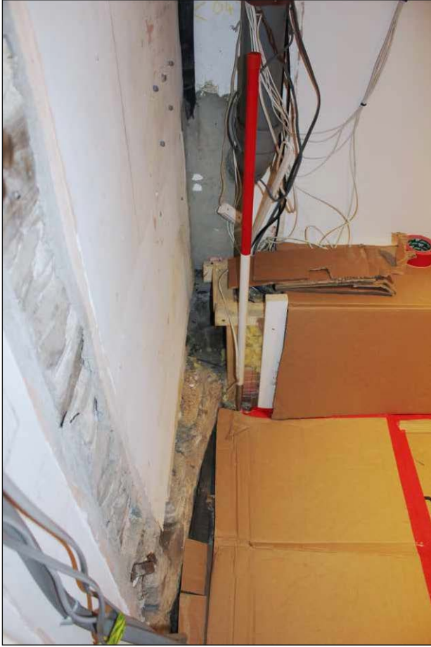
Plate 9: The lower curved masonry of the tide mill, looking northwest (1m scale)
