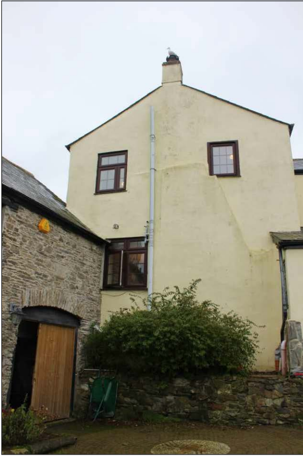
Plate 3: The east elevation of the mill house with the north elevation of the tide mill to the left, looking southwest. In the latter rebuilt masonry is visible above the doorway
