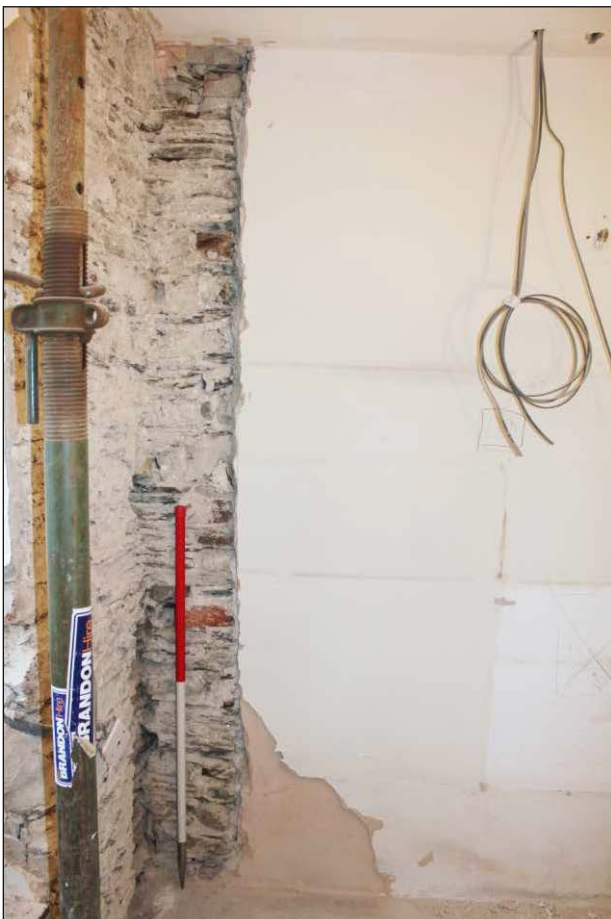
Plate 8: The masonry of the mill house following removal of plaster showing the east edge of a blocked doorway, looking southeast (1m scale)
