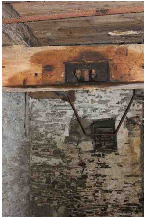
Plate 16: View of end bearing box and other lineshaft brackets at the northeast side of the first floor, looking east
