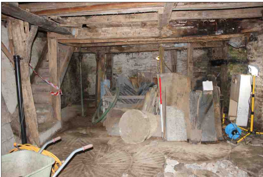
Plate 11: General view of ground floor, with millstones set into the floor in the foreground and north hurst frame to the rear, looking north (1m scale)
