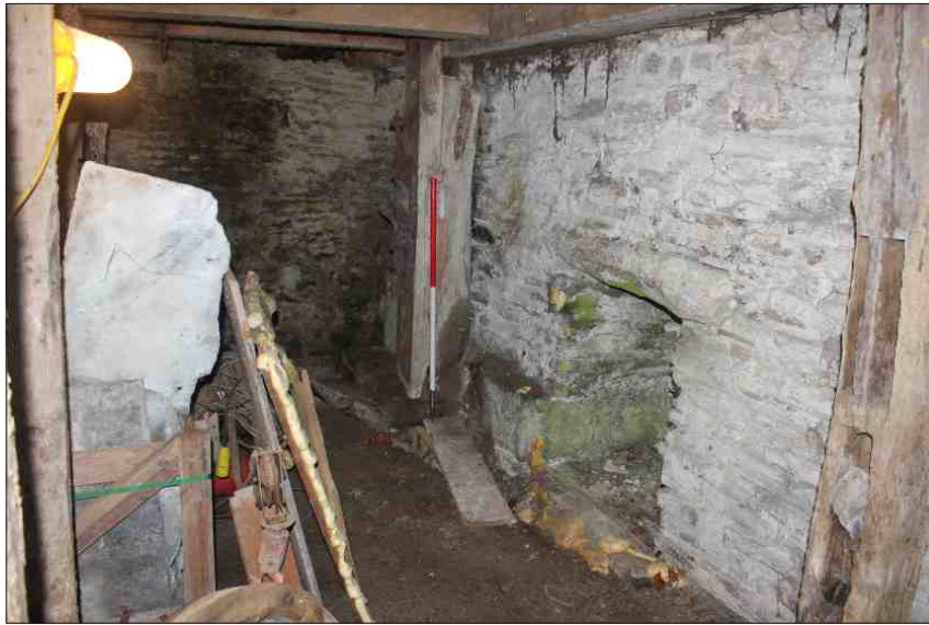
Plate 13: View of wheelshaft hole, hurst frame and fittings at the north end of the ground floor, looking northwest (1m scale)
