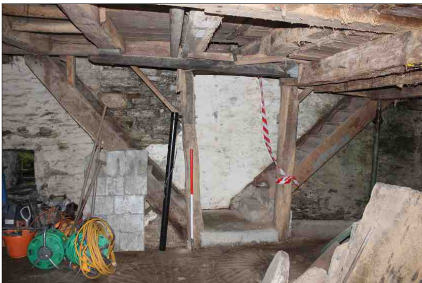
Plate 12: View of staircases on the ground floor with the break in the west wall behind, looking west (1m scale)
