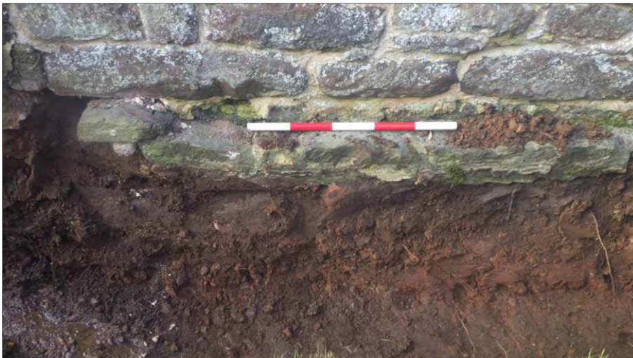
Plate 2: Representation of excavated drain trench with exposed footing S107. Chancel elevation, view to west (scale 0.5m)
