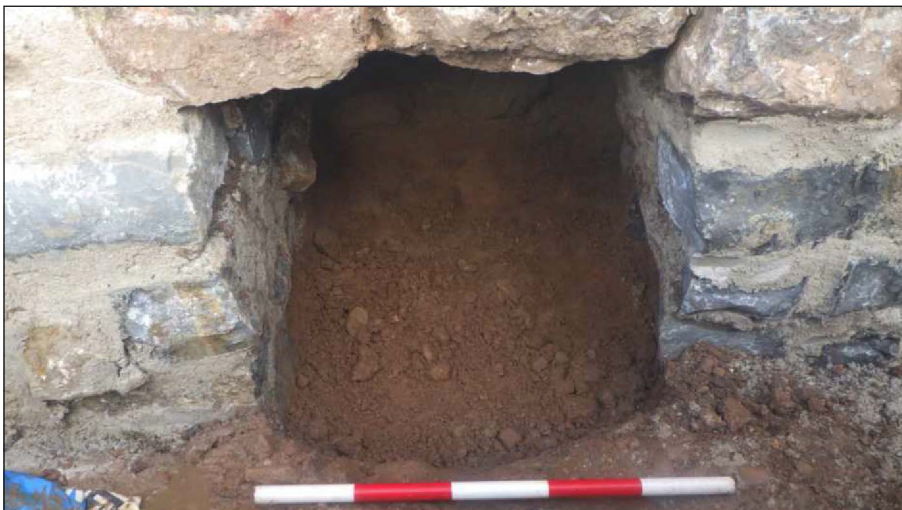
Plate 3: Showing underpinning pit excavated into chancel wall footing. View to north (scale 0.5m)
