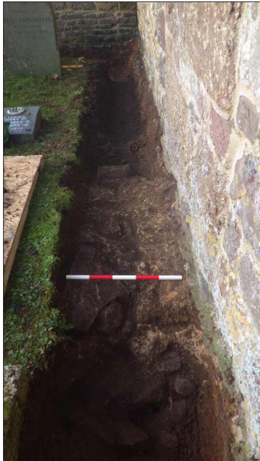
Plate 4: Showing excavated drain trench with footing S103. View to west (scale 0.5m)
