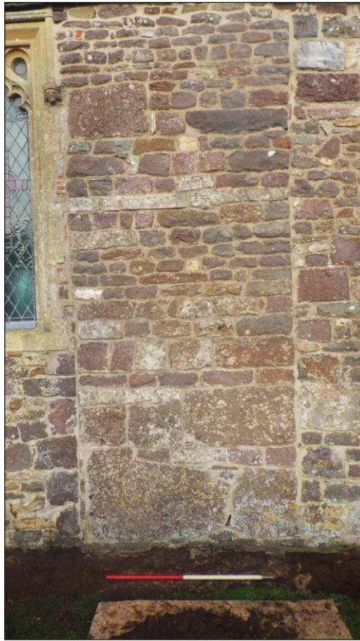
Plate 6: Plate 6. Showing footing S103 in relation to masonry scar of former rood screen stair turret. View to north (scale 1m)
