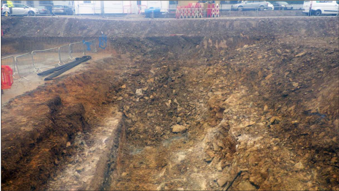
Plate 5: The Dock Lines ditch (part backfilled) during bulk reduction, looking northeast. (1m scale)
