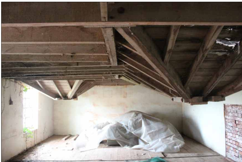
Plate 3: Unit 1, the hoppers extending down from the second floor to the first floor, looking southeast
