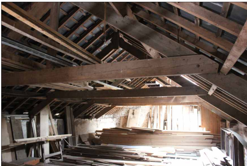
Plate 6: Unit 3, the first floor showing the roof structure supported on the south elevation, looking southeast
