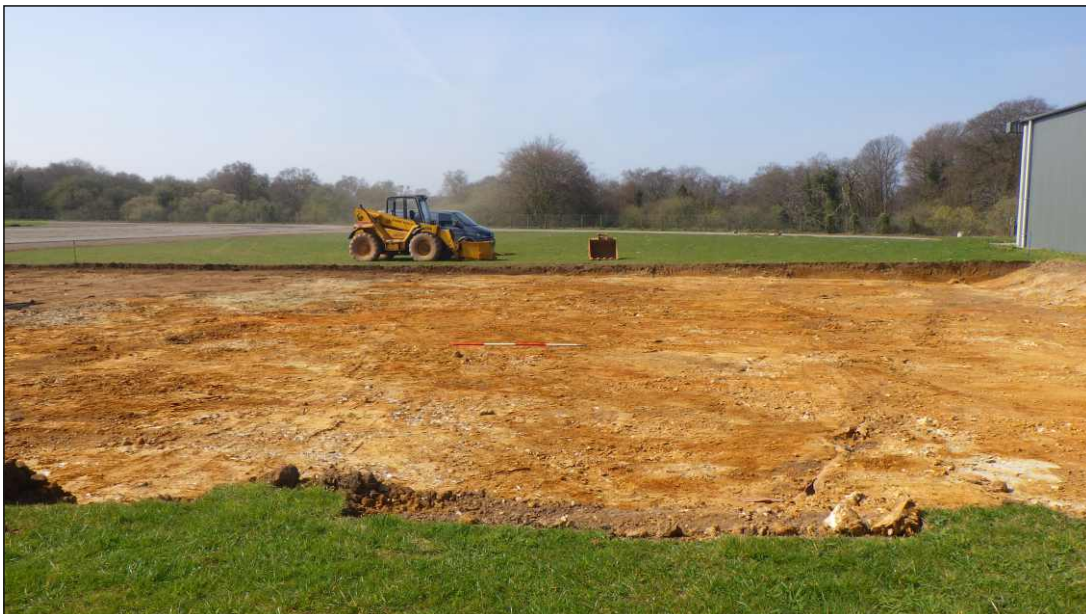
Plate 4: Area following ground reduction, looking west, showing patches of flint and chalk bottom right and top left (2m scale)
