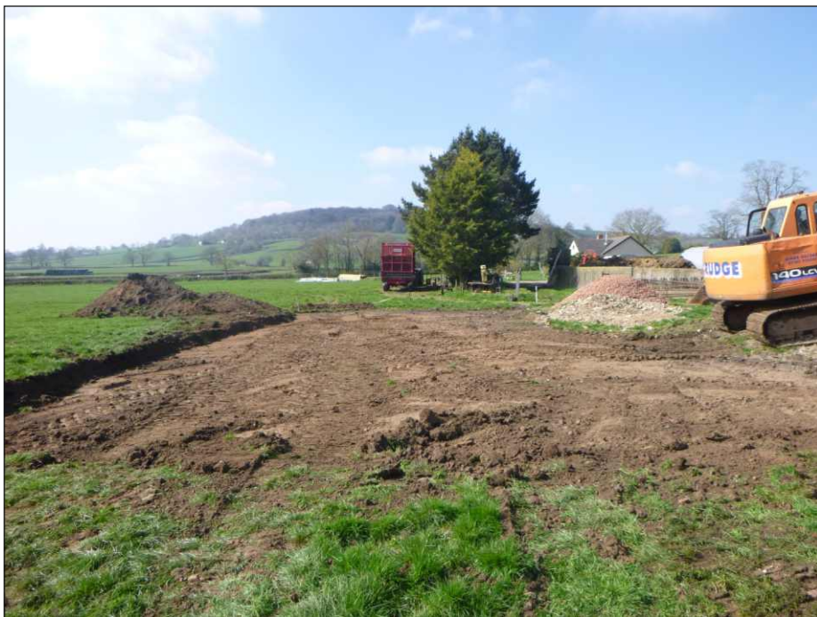
Plate 2: General view of the monitored area following stripping, view to the west
