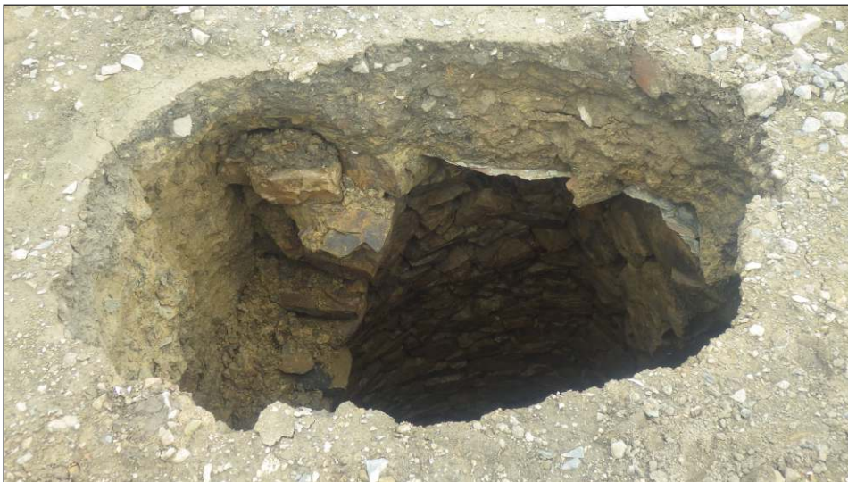
Plate 2: The well showing stone lining and collapsed slate covering, looking south
