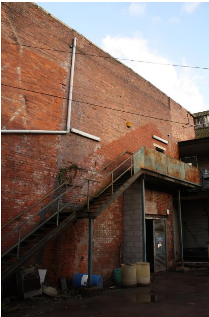
Building 21 Compressor Room, south elevation facing north-east. The gable of an earlier, lower building can be seen which is similar to another gable within the wall of the Reactor Room to the west, illustrated below. (8340)
