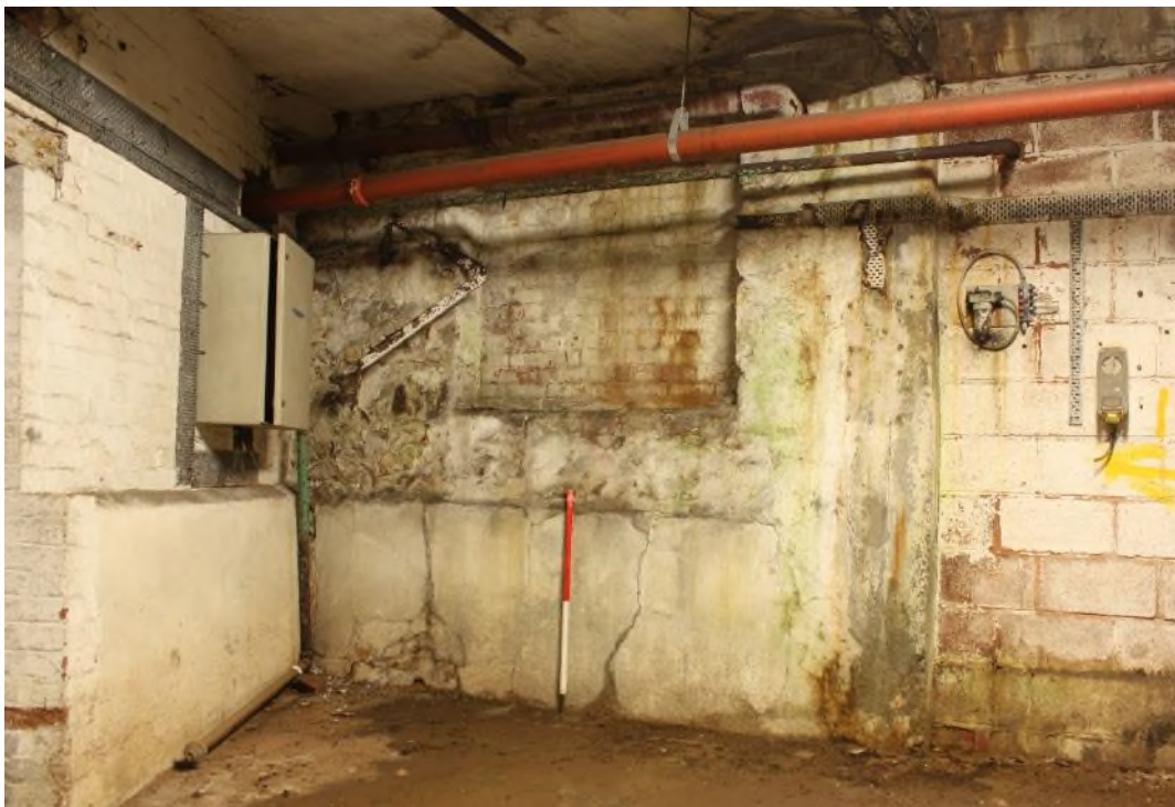
Building 15 North-east wall of the former angled range built between 1842 and 1879 showing an element of stone rubble masonry at the north-west end. Facing north. (9436)
