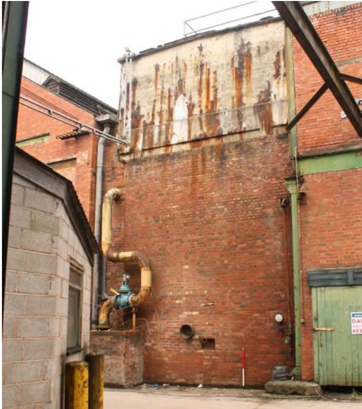
Building 20, south elevation, east part showing the later infill section with a tank on the flat roof. (9534)
