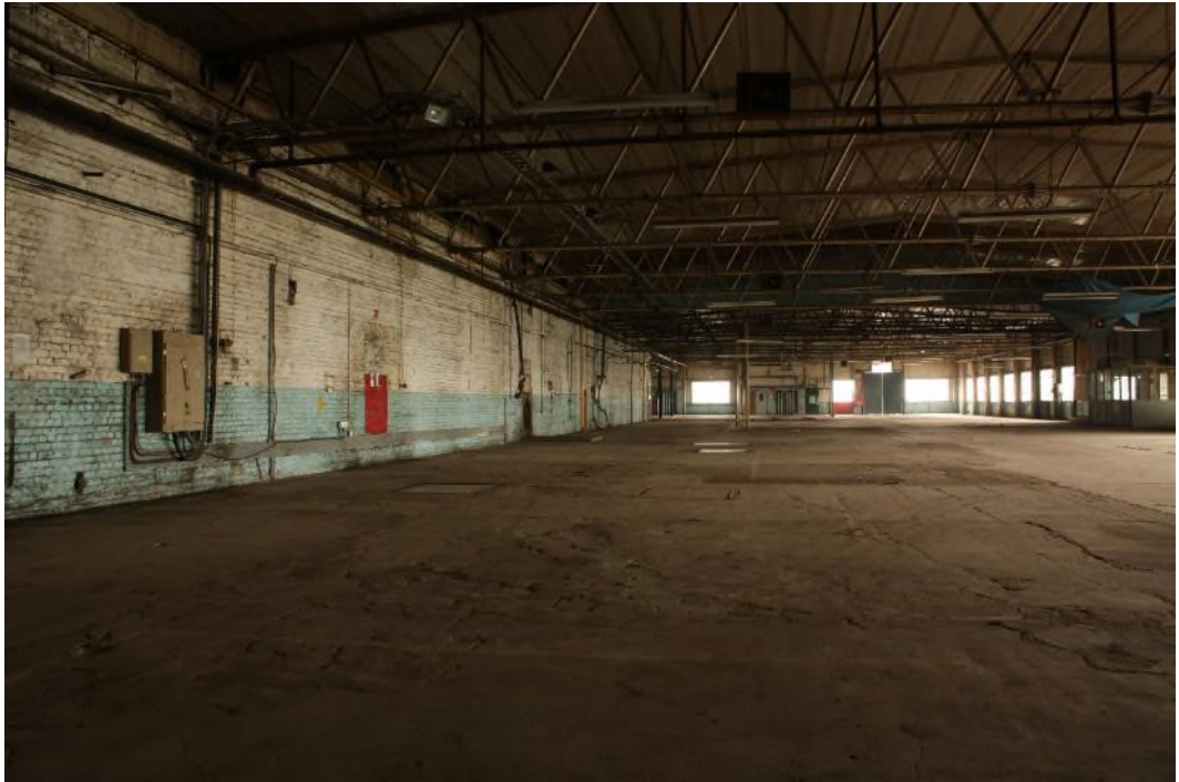
Building 3 Upper floor facing west-south-west to the south wall of the building. (9574)
