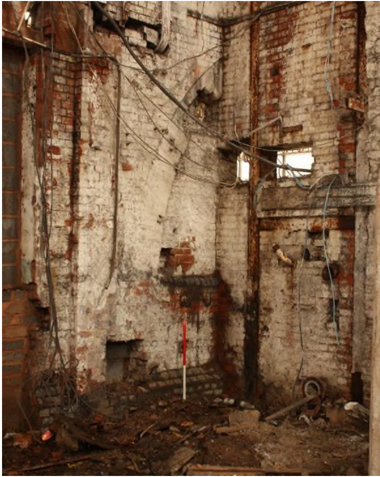
Building 22 North-west corner of the Reactor House showing the arch cut by the north wall of Bdg. 22. (9545)
