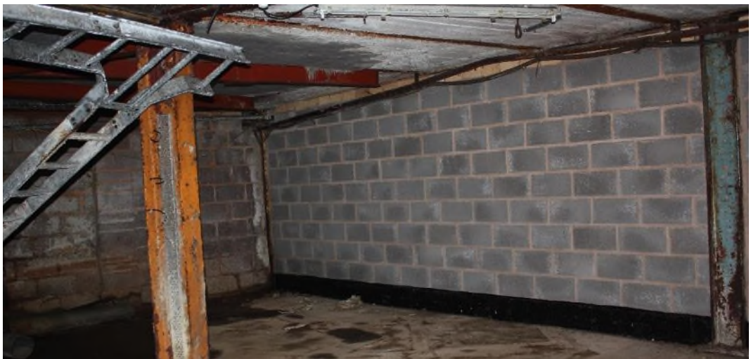
South part of the area of Building 14 with modern blockwork wall dividing the space. (8116)
