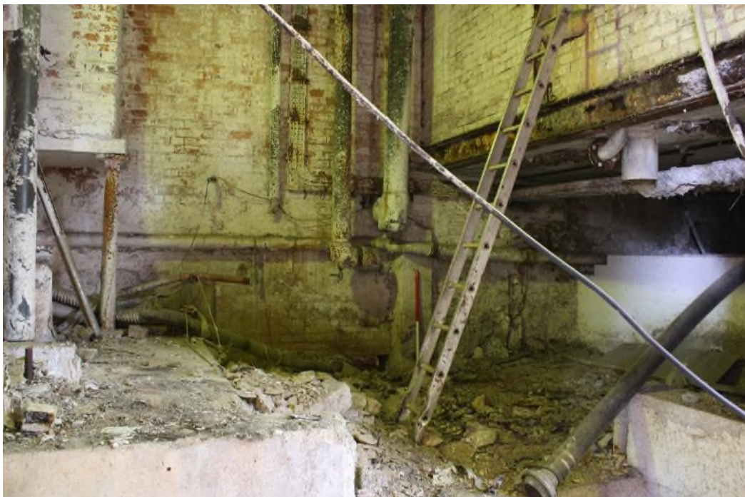
Interior of the Pump House, south part facing north-west – the turbine pit is located beneath the jettied structure, top right. (9514)
