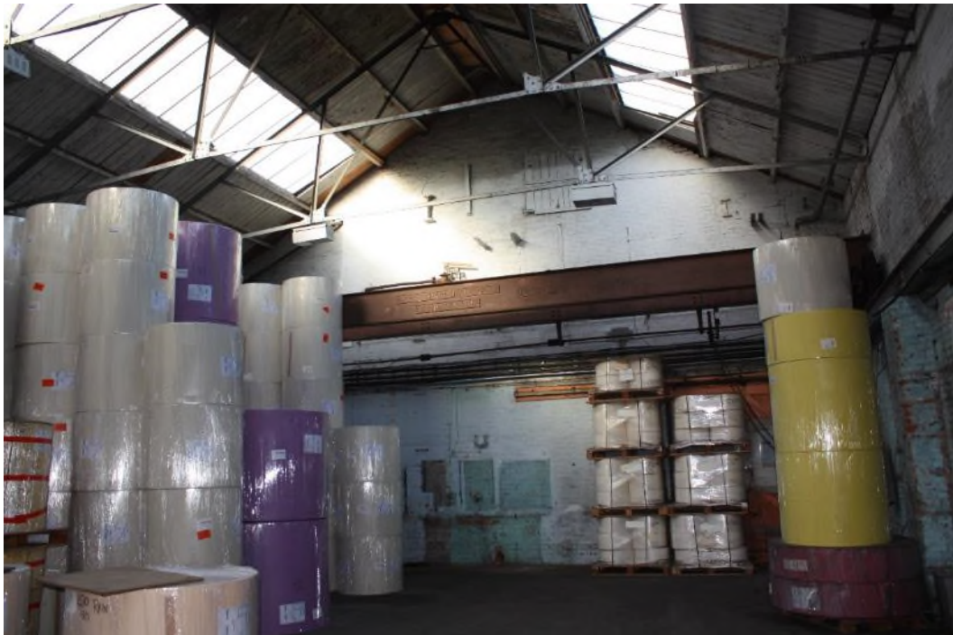
Building 28 Interior facing north showing the crane running on rails against the side walls. (8368)
