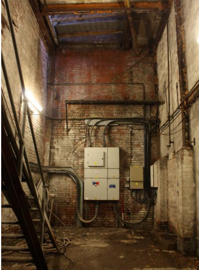
Building 10 North wall of the Grass Boiler Room showing blocked arched window.
