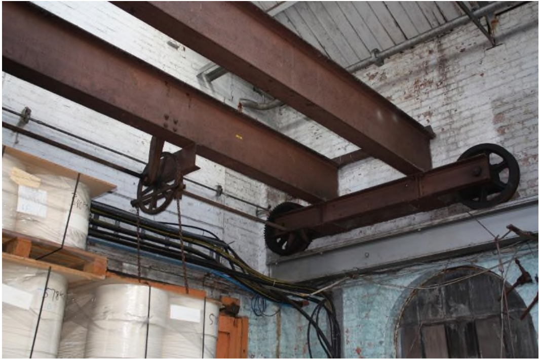
Building 28 Travelling hoist.
