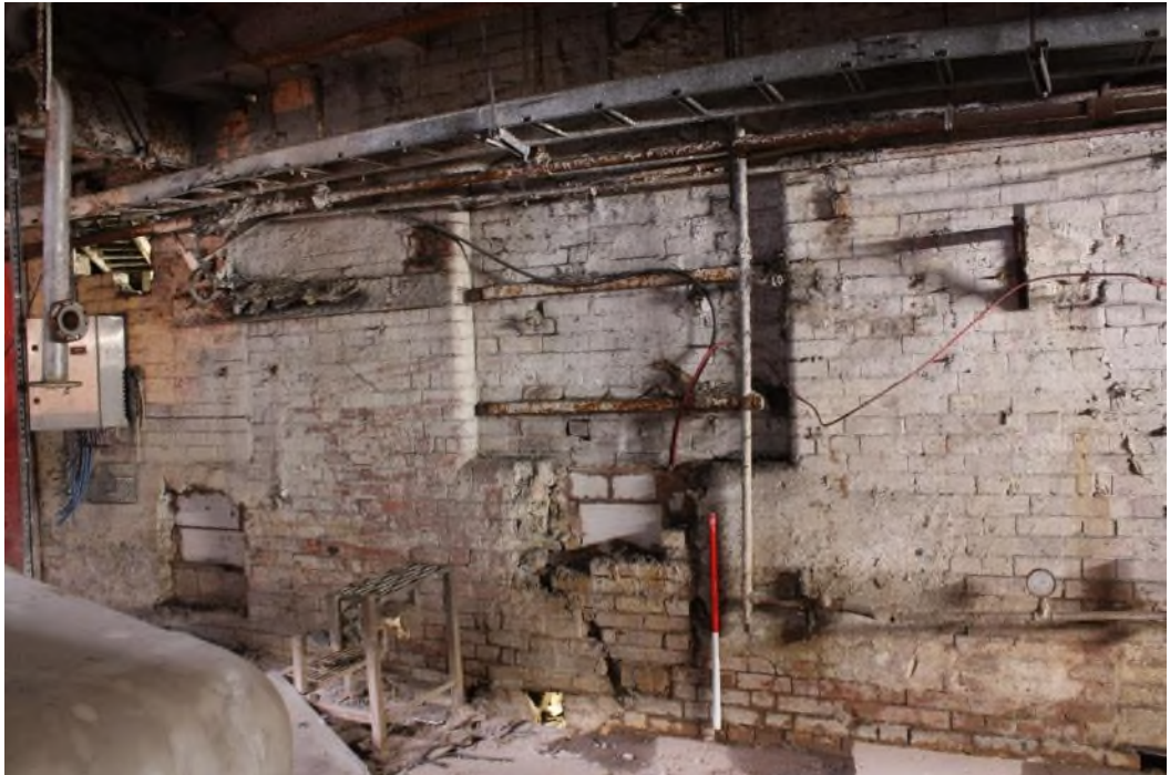
Building 16 South elevation facing into gap between Bdg. 16 to the north and Bdg. 23 to the south showing one of several blocked windows. Facing north. (9491)
