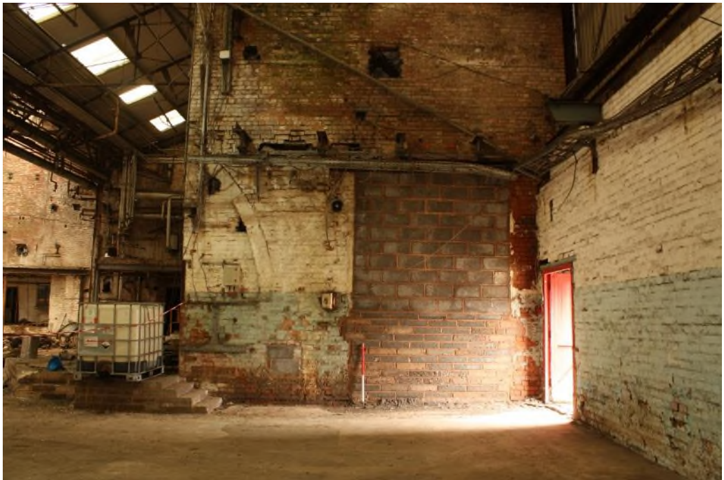
Building 22, west wall showing the partial arch taken from within Bdg. 23, facing south-east. (9550)
