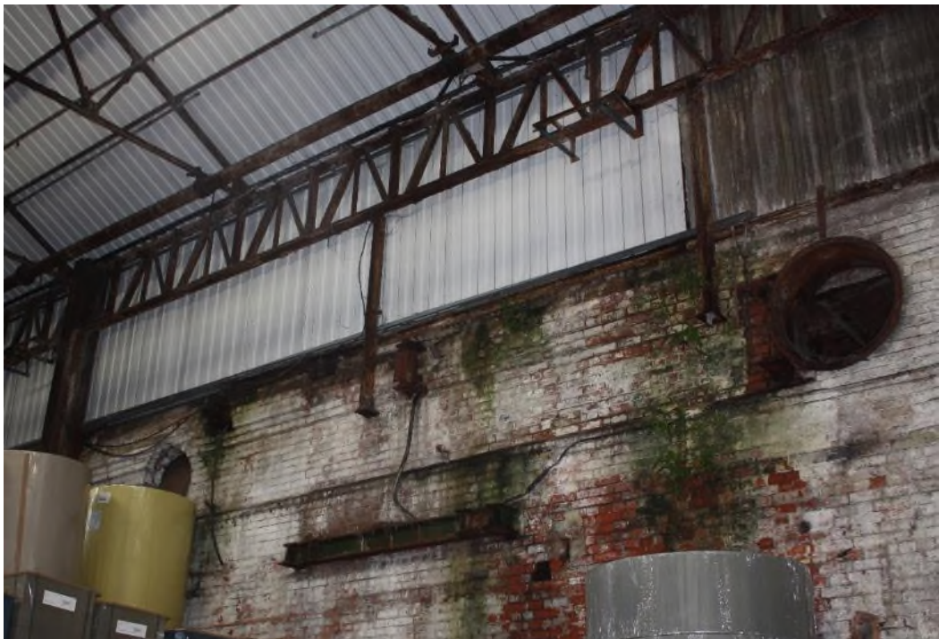
Building 23 Interior, north wall, central section facing north-west showing circular openings in the upper part of the wall. (8336)
