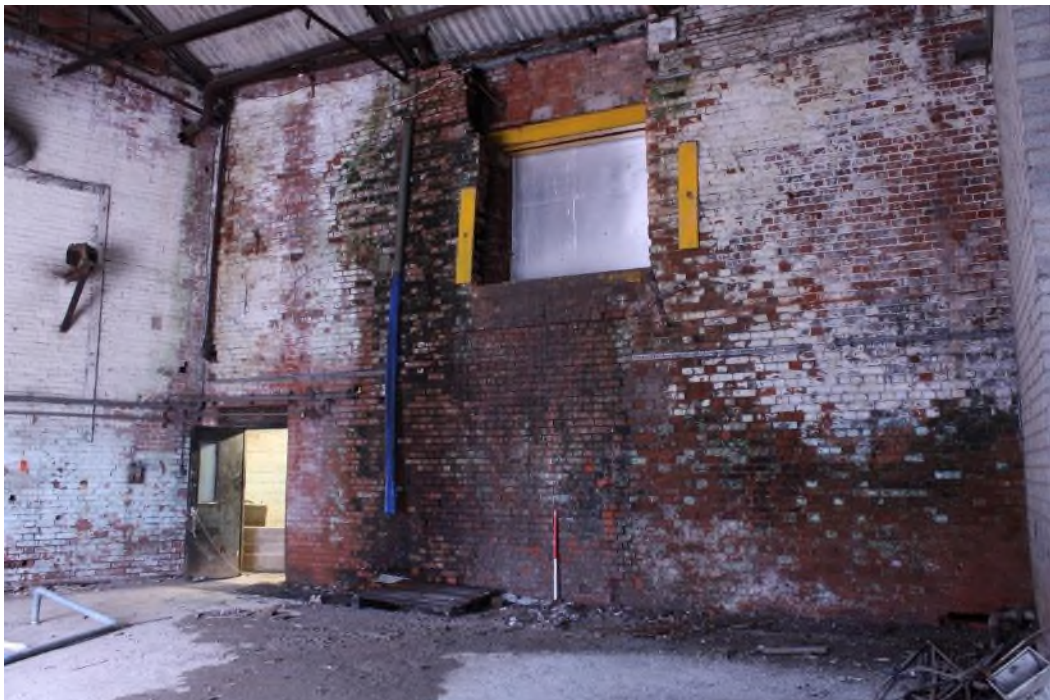
Interior of Building 8, south wall. The double skin of brickwork can be seen above the large opening at higher level. (9582)
