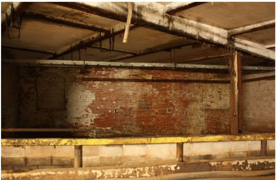
Building 16 South-east wall, inner face (north-west) showing blocked window openings. Facing south-east. (9478)
