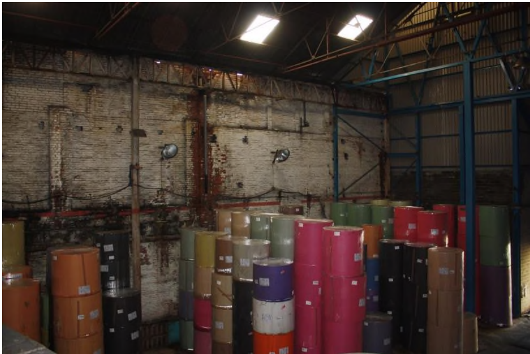
Building 22 Interior of the Reactor House taken from the upper level within Bdg.21, facing south-west. (8353)
