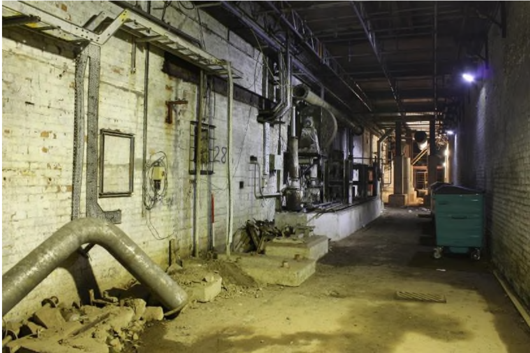
View along the Tunnel Passage to the west. The north wall of Bdg.6 is to the left and the south wall of Bdg.3 to the right. (9586)
