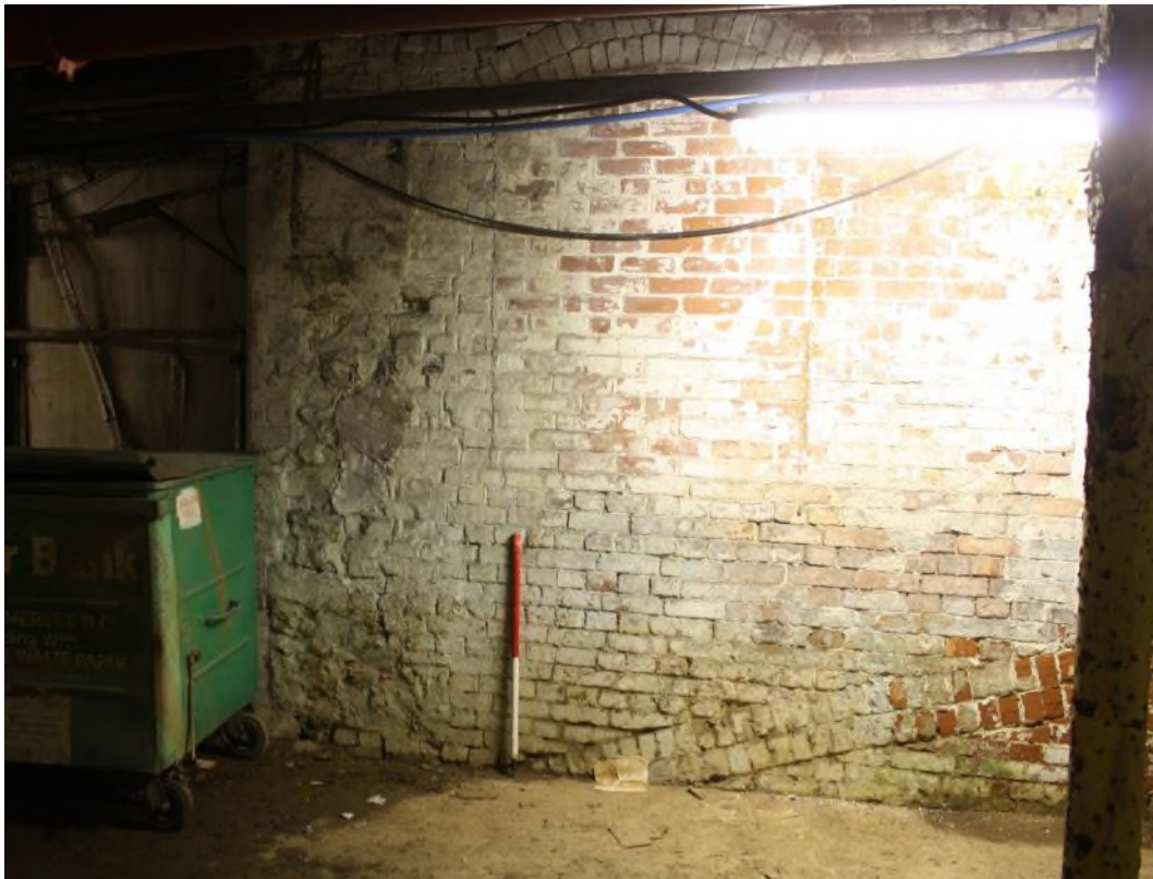
Building 16 The south end of the east wall is showing an area of rubble stonework, the beginning of the low arch spanning the river and a blocked window. Facing west. (9548)
