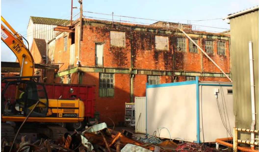
Building 19 The Compressor Room is located in the lower left had part of the east elevation of this large building which includes the Power House Bdg. 20. (8080)
