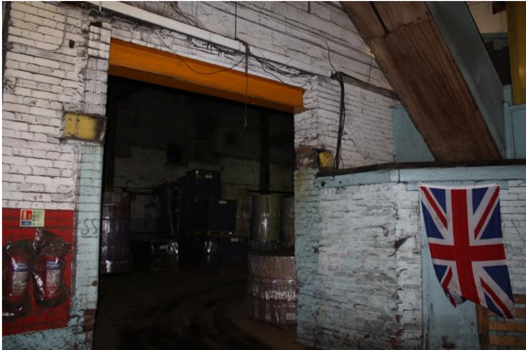
Building 23 Interior, north-west corner looking north into Bdg. 6. The brickwork of an arch-headed window can be seen to the right of the inserted opening. At the higher level the wall is constructed in blockwork.
