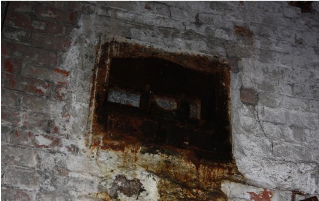
Figure Drive shaft bearing in the west wall of the northern part of the Pump House (8499).
