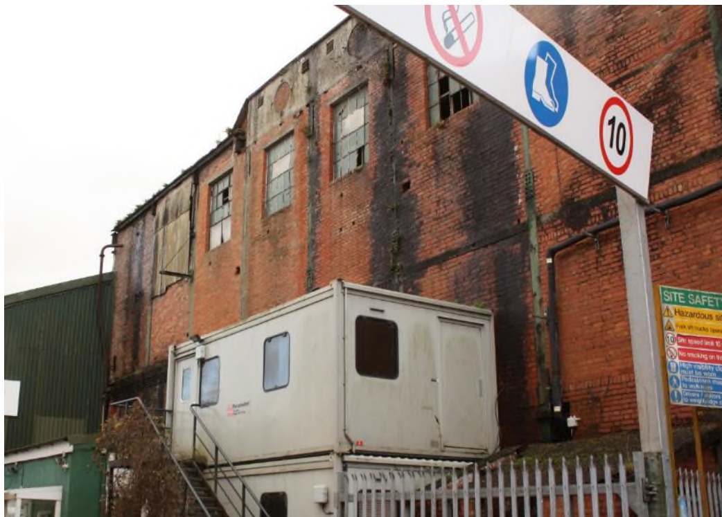
The north elevation above Buildings 9 and 10 with the modern green metal clad steel-framed Building 11 just visible to the left of the picture. (8284)
