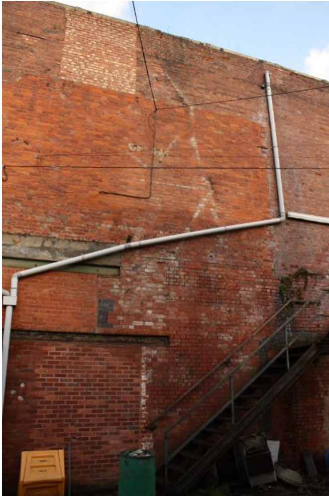
Building 22 Reactor House, south elevation, east part facing north-east. This shows a much altered brick elevation with a vertical joint in the brickwork to the left of the downpipe. (8339)
