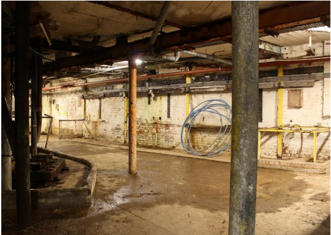
Building 15 North-east wall of the former angled range, originally built between 1842 and 1879 although the present wall may be a later rebuilding. Facing north. (9427)
