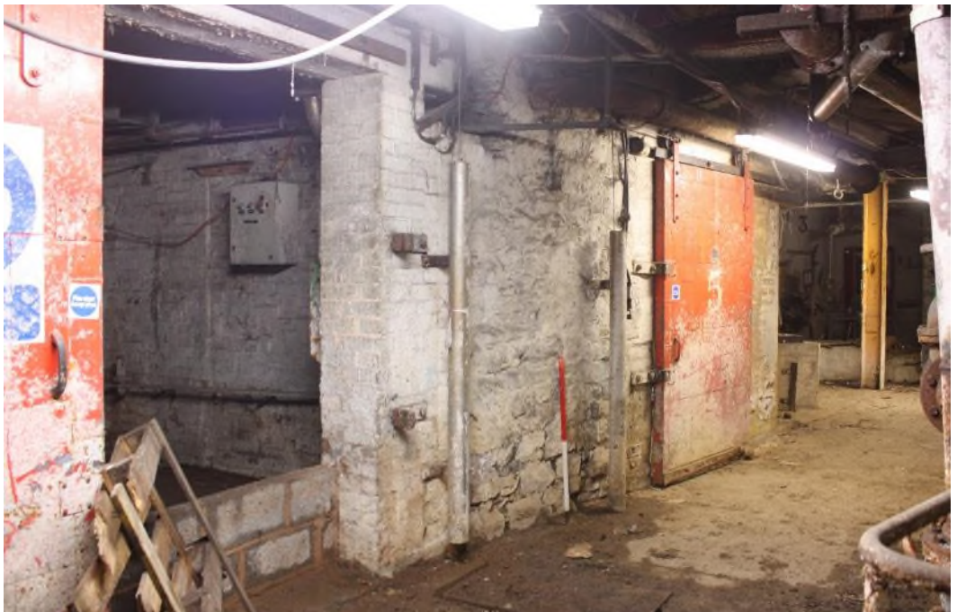
Building 16 South end of the north range showing a section of stone rubble walling in the south-east wall. The corridor to the right of the picture is a gap between Bdgs. 16 and 15. (9486)
