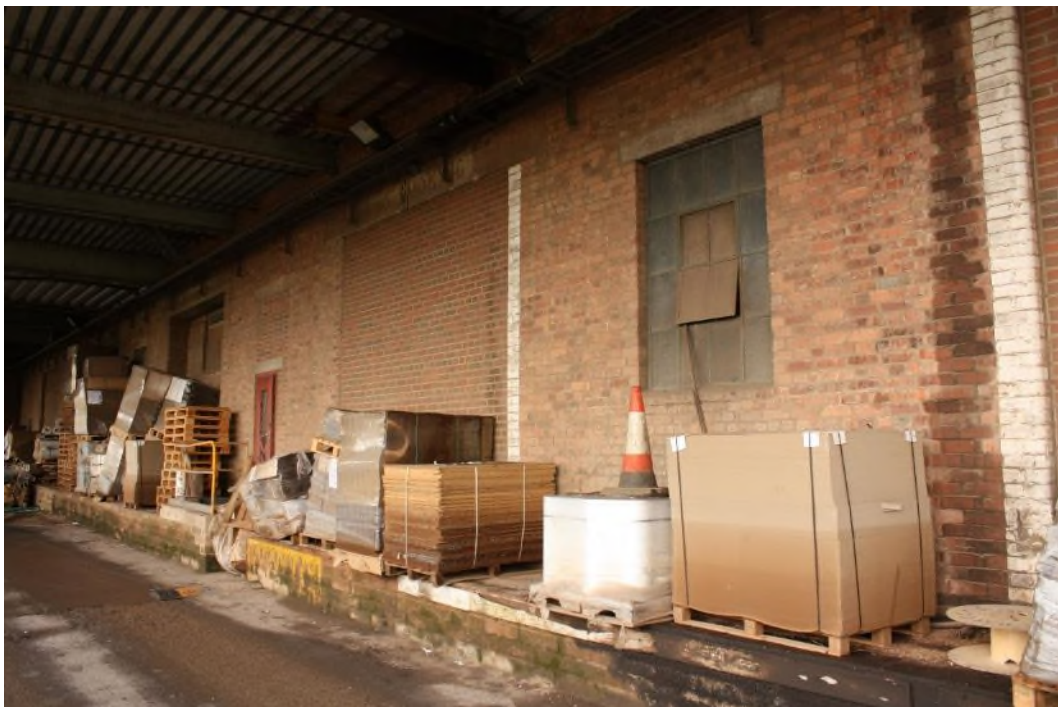
Building 3 North elevation – probable earlier (but probably post 1904) section of the north wall beneath Covered way, facing south-east. (8285)
