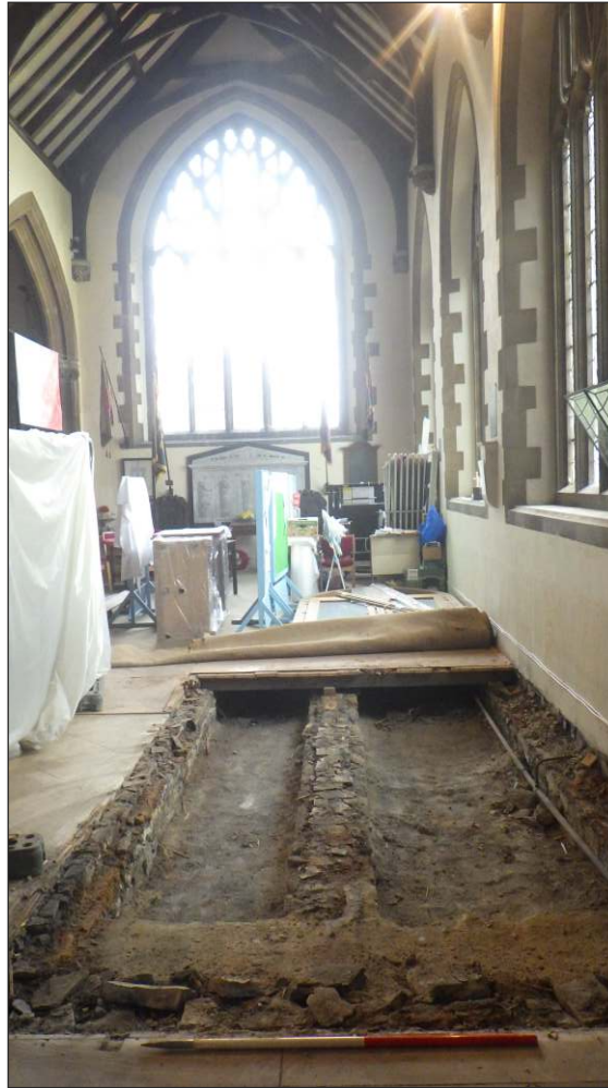
Plate 2: Showing area of removed timber support plinth with exposed sleeper walls below. view to east
