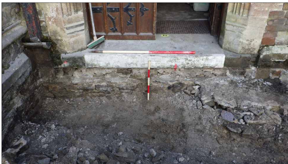
Plate 3: Southeast end of the drain trench, looking south (1m and 0.5m scales)
