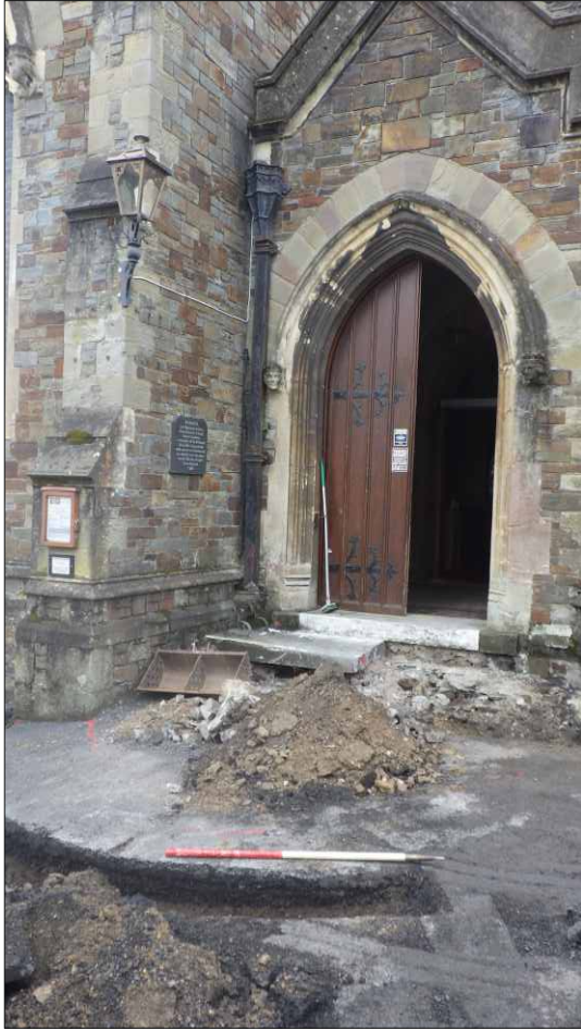
Plate 1: General view of the monitored works area with the steps trench in the foreground, looking southeast (1m scale)
