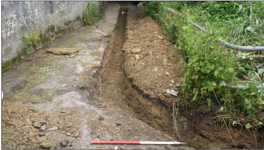
Plate 7: View of the east end of the trench in the embankment, looking west (1m scale)
