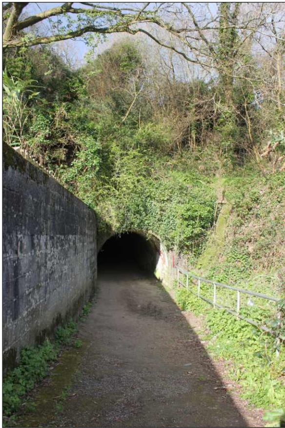
Plate 1: Pre-works view looking west across the embankment towards the east portal of the tunnel (1m scale)
