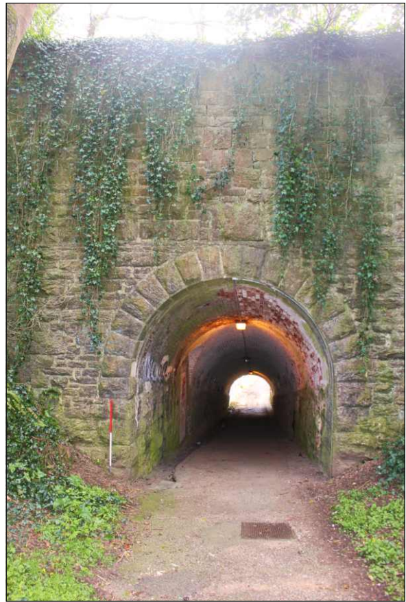
Plate 2: Pre-works view looking east down the cutting into the west portal of the tunnel (1m scale)
