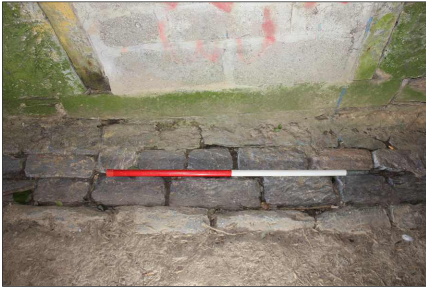
Plate 4: Close-up view of the historic drain in front of the western blocked doorway, looking north (1m scale)
