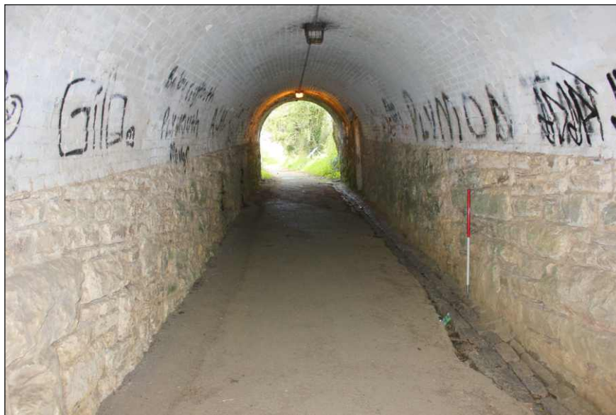
Plate 3: Pre-works view looking east through the tunnel showing the brick arch, the modern surface with earlier drain to the right, and the western blocked doorway (1m scale)
