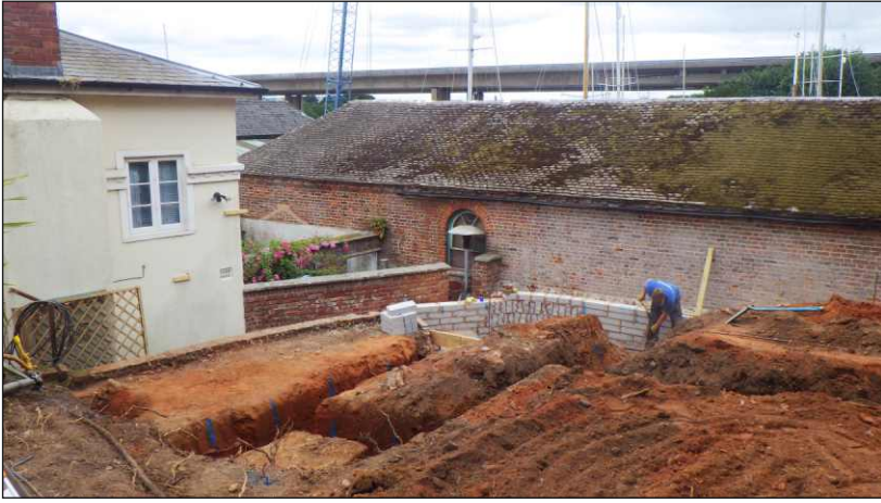
Plate 1: General view of site looking west towards Reeds and Retreat Boat Yard
