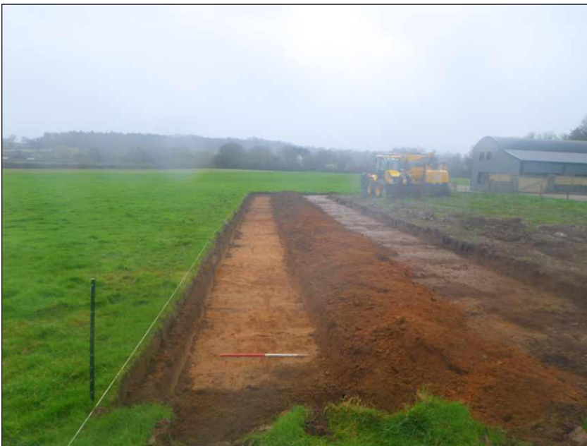
Plate 2: Showing drainage trench along east side of site. View to south (scale 1m)
