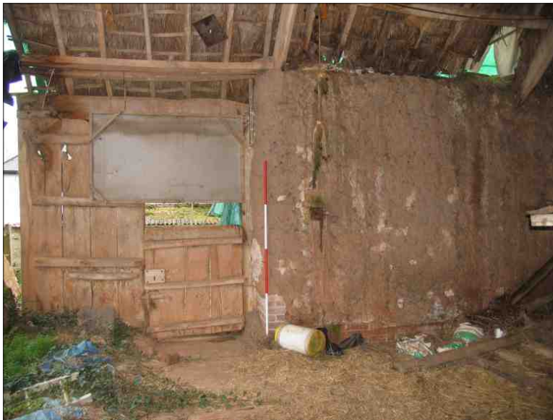
Plate 11: Double doors in the south elevation of the threshing barn, looking south (2m scale)
