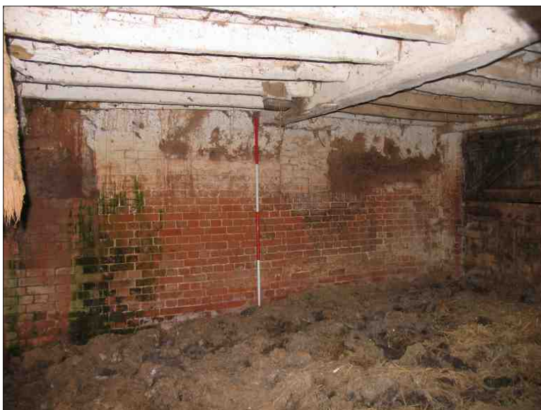
Plate 12: The stable within the threshing barn showing the blocked window in the west elevation, looking west (2m scale)
