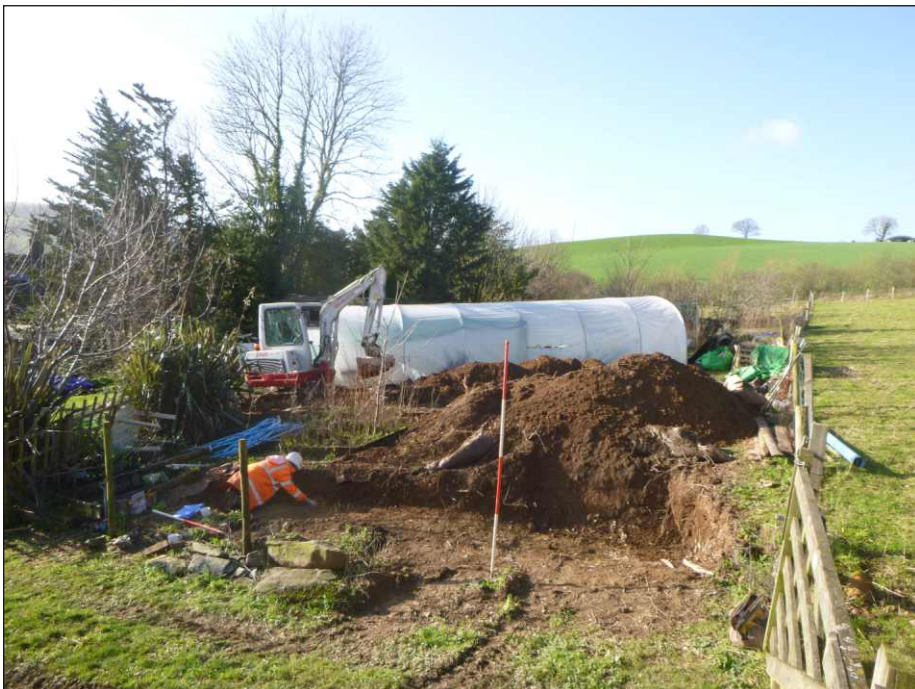
Plate 2: General working view of site, looking west with Trench 2 in foreground (scale 2m)
