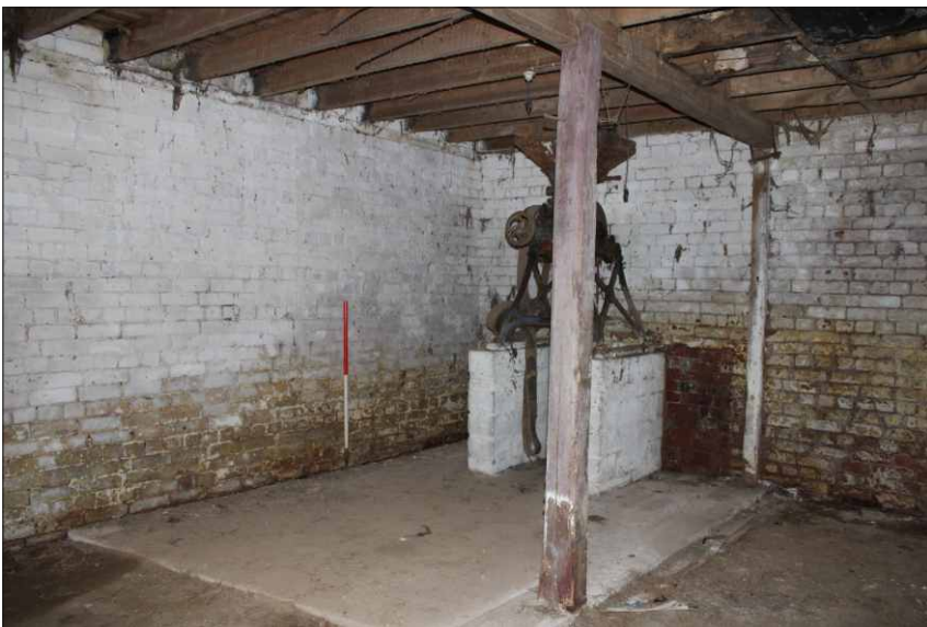
Plate 5: Internal view of south end of the stables, looking southwest (1m scale)
