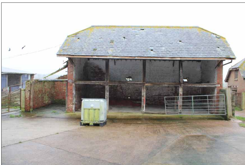
Plate 21: West elevation of the bottom cattle building and the store, looking east (1m scale)
