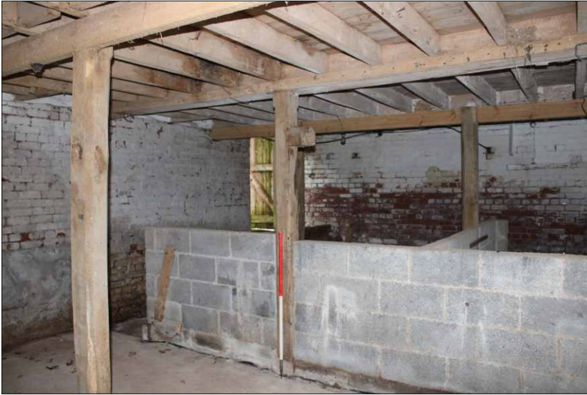
Plate 4: Internal view of north end of the stables, looking northwest (1m scale)
