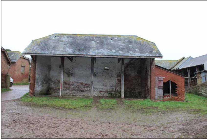
Plate 19: East elevation of cart linhay and brick shed, looking west (1m scale)
