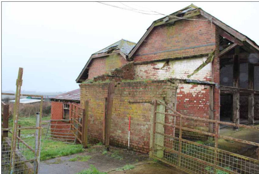
Plate 20: North elevations of the bottom cattle building, the cart linhay, brick shed and store, looking southeast (1m scale)
