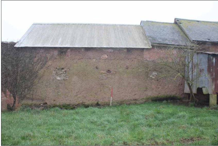
Plate 13: North elevation of the far side cattle building, looking south (1m scale)
