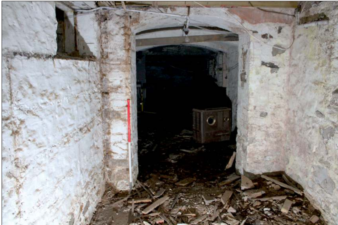
Plate 7: The north rooms with vaulted ceilings in the basement, looking south (1m scale)
