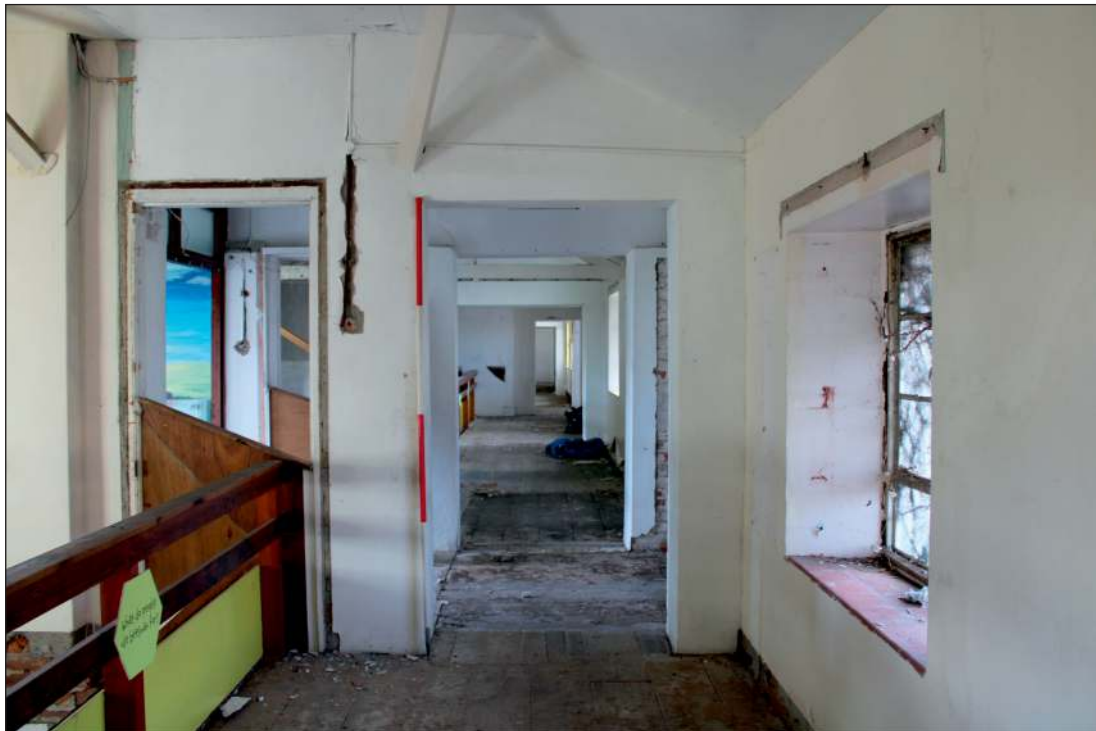
Plate 14: General view of the first floor of the central range showing the walkway and viewing platform, looking west (2m scale)
