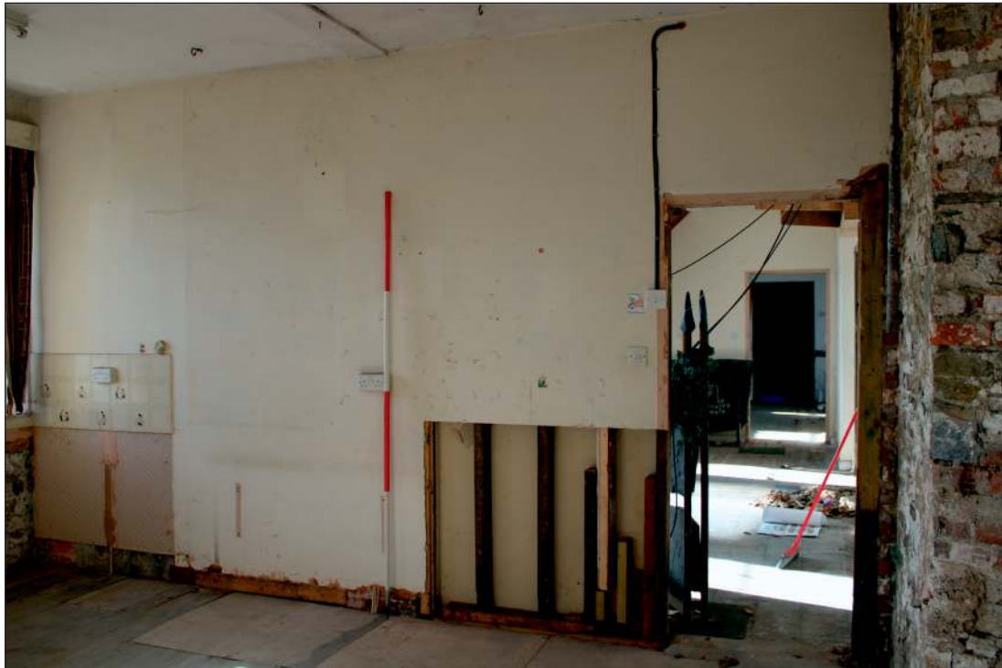
Plate 5: The east partition to the entrance hall of the south range, looking west from the adjacent room (2m scale)
