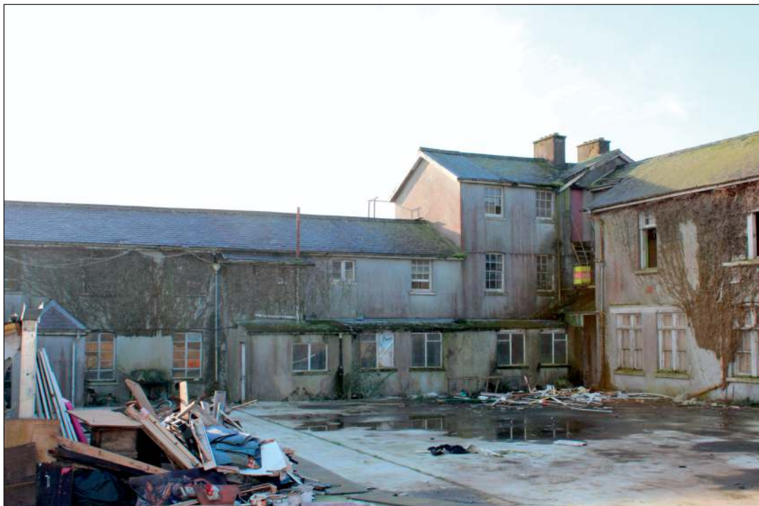
Plate 10: The north elevation of the central range, east section looking southwest also showing the south end of the north range
