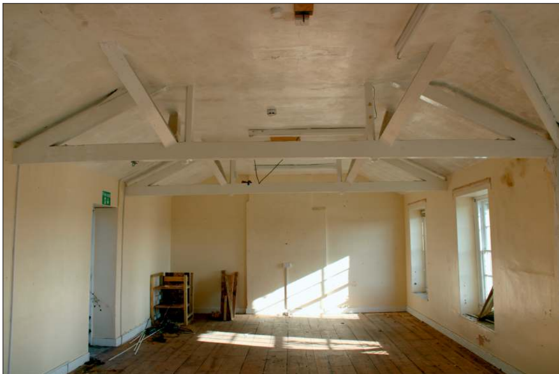
Plate 6: The first floor of the south range, looking east showing the roof structure
