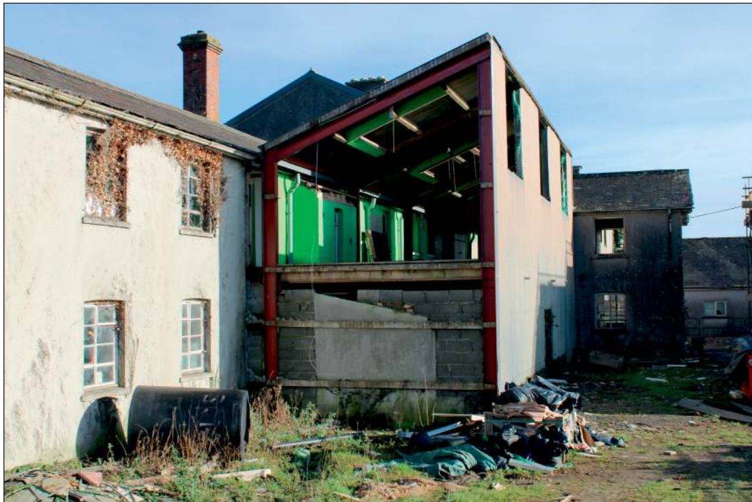
Plate 8: The south elevation at the west end of the central range showing 1970s addition and link to the south range beyond, looking east
