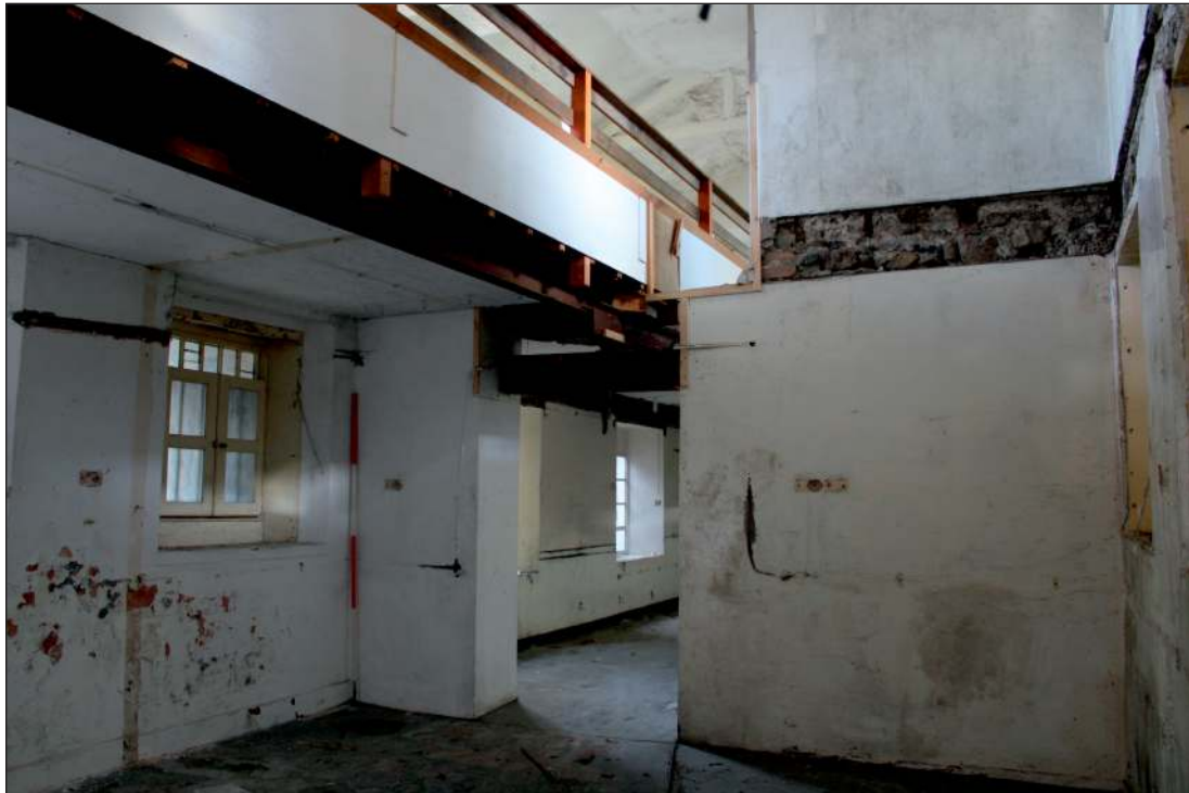
Plate 13: Central and eastern rooms in the central range, showing barred window and replaced first-floor structure, looking northeast (2m scale)
