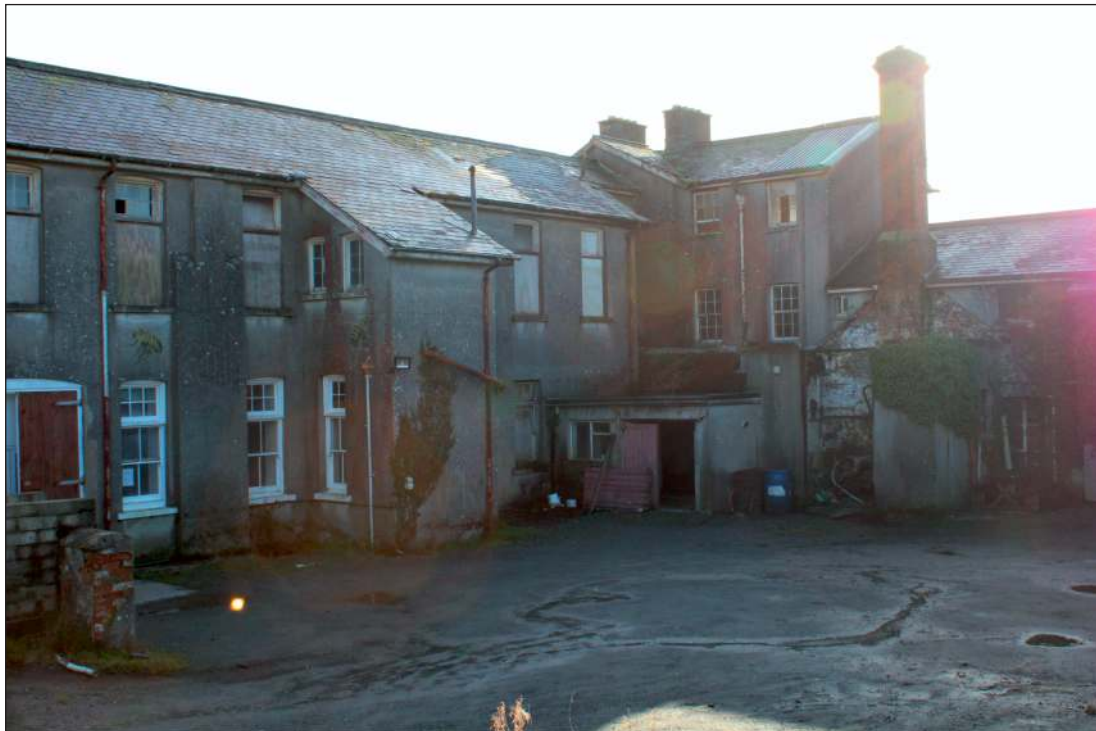
Plate 20: The west elevation of the north range, southern section showing integral service tower and later extensions, looking southeast
