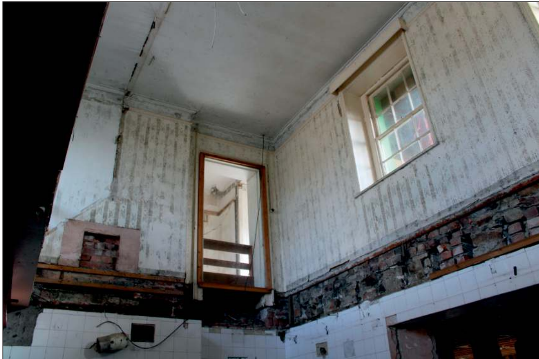
Plate 15: The central western first-floor room of the central range, looking southeast up from the ground floor showing fireplace, cornice, picture rail and sash windows
