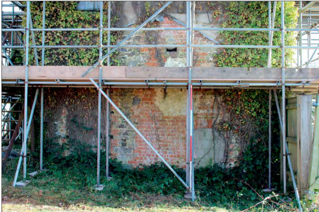
Plate 3: The west elevation of the central section of the south range, looking east showing blocked openings and roof scar (2m scale)
