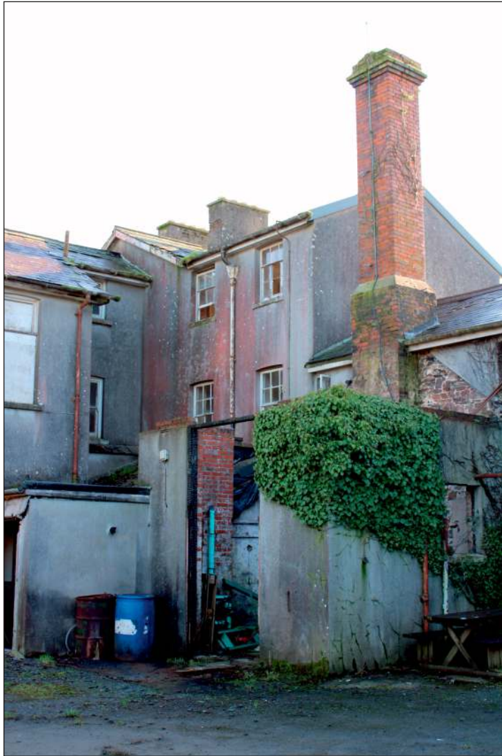
Plate 9: The north elevation of the central range, west section looking southeast showing boiler room and kitchen extensions with the taller central section beyond
