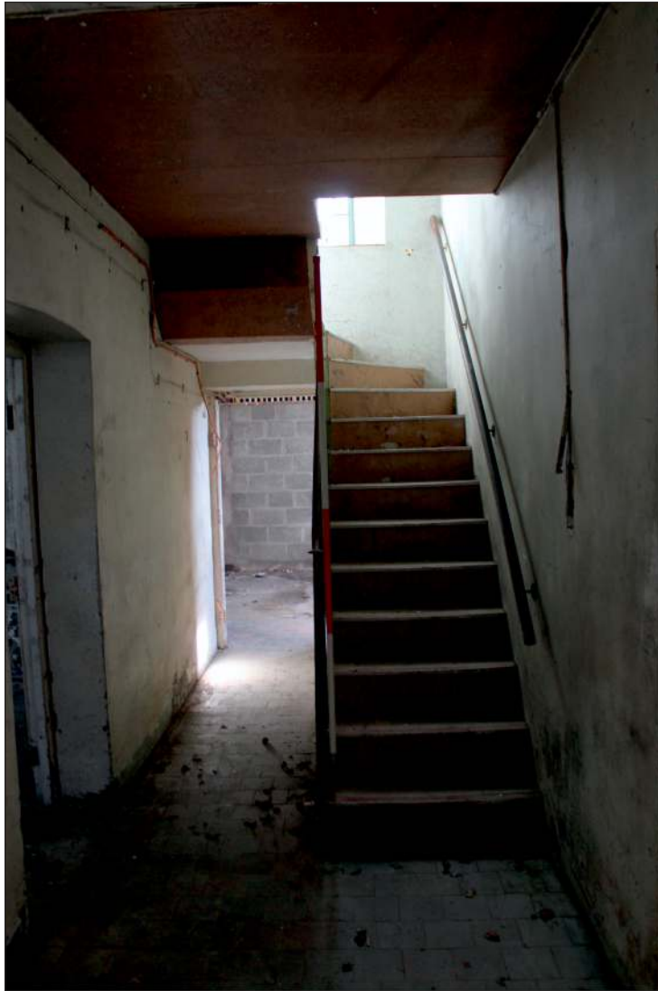
Plate 11: The passage and staircase in the west side of the central range, looking south (2m scale)
