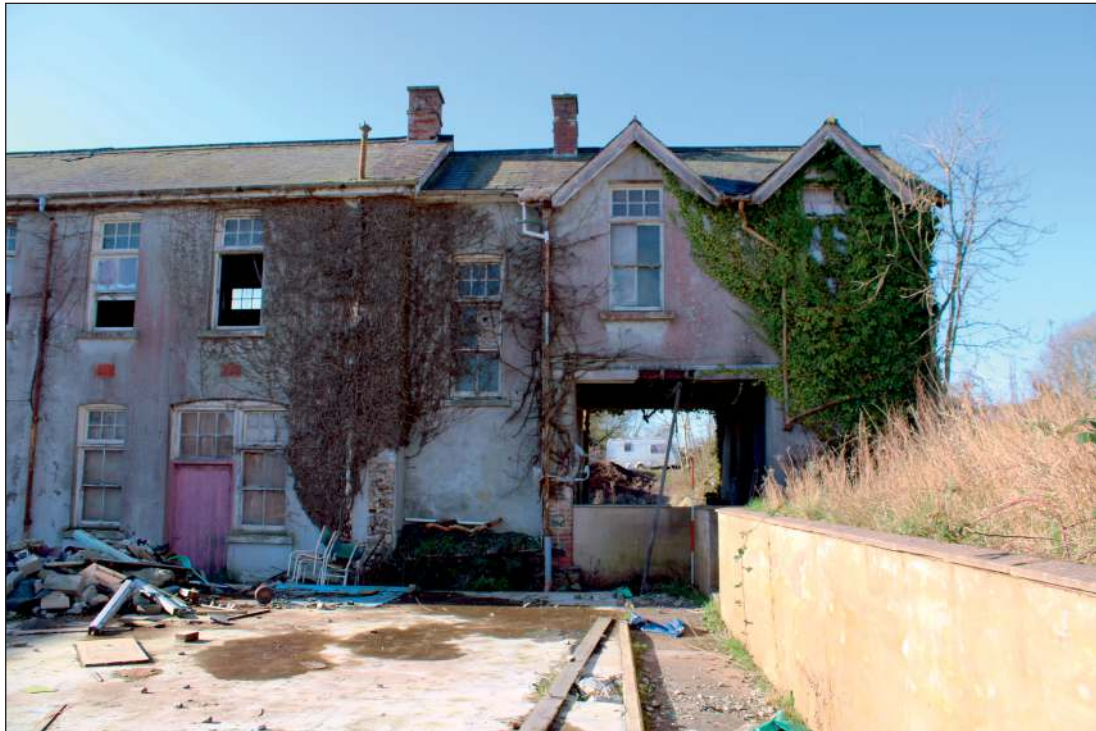
Plate 19: The east elevation of the north range, north end, looking west showing passageway with scar of original yard wall to left of scale (2m scale)
