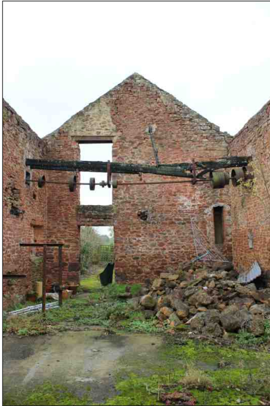
Plate 10: The west end of the threshing barn showing openings, overhead lineshaft, and evidence for a partial first floor, looking west
