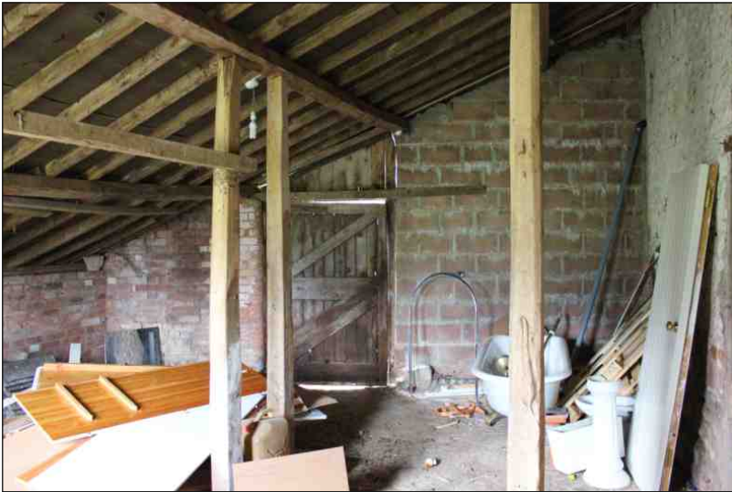
Plate 8: The interior of the brick extension to the east range, showing the east elevation and vertical posts, looking west
