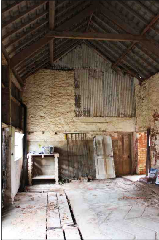
Plate 4: The north end of the east range, showing various openings, the floor, evidence for the former first floor and the roof structure, looking north
