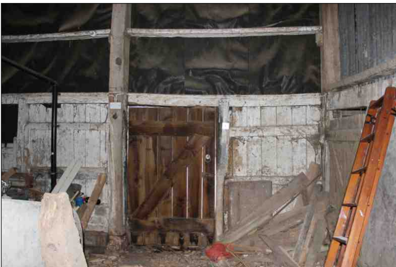
Plate 3: The interior of the east range showing the primary finish of the west elevation, looking west
