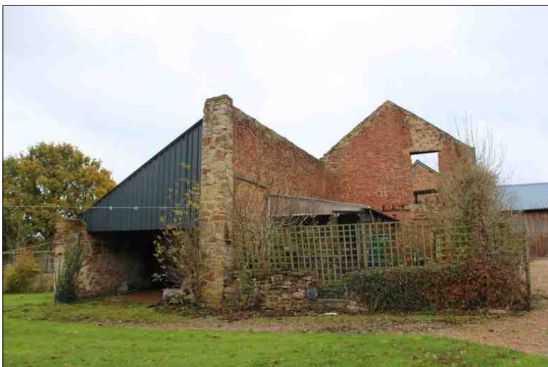
Plate 12: The west barn in the north range and attached implement shed, looking northeast
