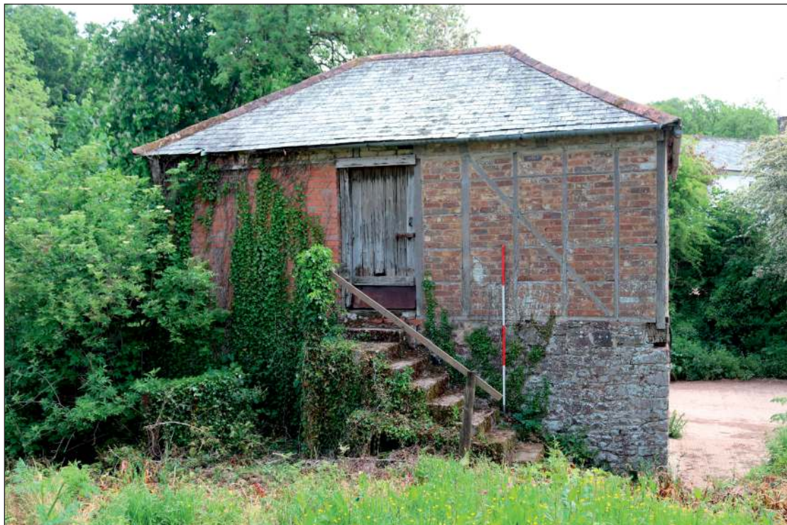
Plate 4: The west elevation looking east, showing the steps to the first floor, and the replacement brickwork and timber framing (2m scale)
