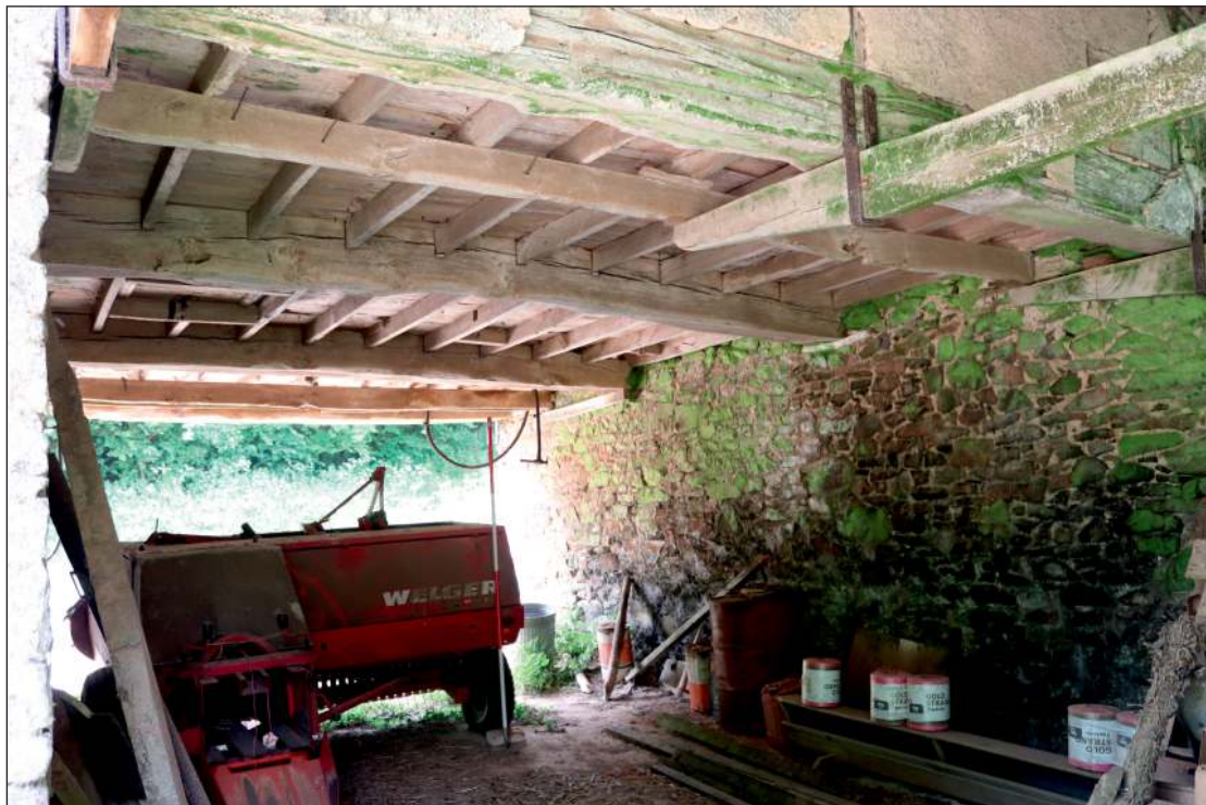
Plate 6: The interior of the ground-floor cart shed looking southwest, showing the hatch (left), bridging beams for the first floor, and brackets and associated secondary beam for the north canopy (2m scale)
