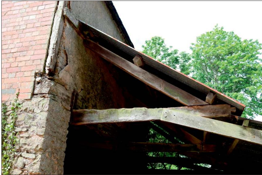
Plate 5: Close-up view of the north canopy looking east, also showing the lath and plaster on the bridging beam for the first floor
