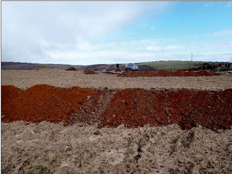
Plate 1: General view of the site with Trench 1 in the foreground, looking northwest
