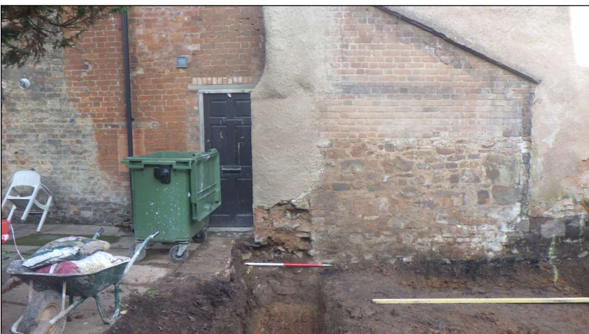
Plate 4: Stone wall foundation S104, showing wall of No. 18 Fore Street above (1m scale)
