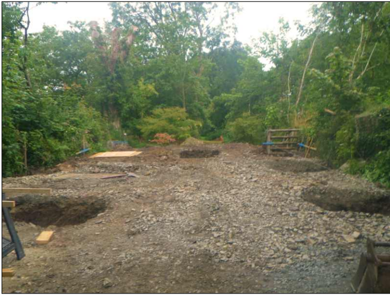
Plate 2: Showing new garage area with excavated foundation pad pits. View to west
