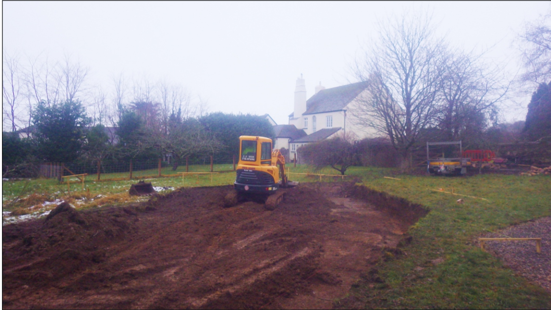
Plate 1: General view of the site, work in progress, looking northwest with Rosemount behind
