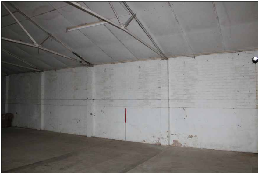
Plate 8: Blocked windows in the west wall of the institute and NAAFI, looking southwest (1m scale)
