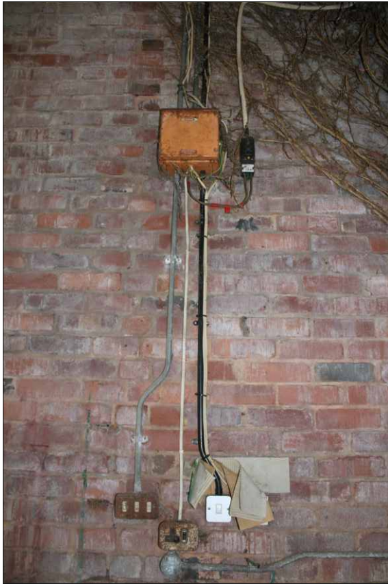
Plate 13: View of electrical fittings on the south wall of the Romney hut, looking south
