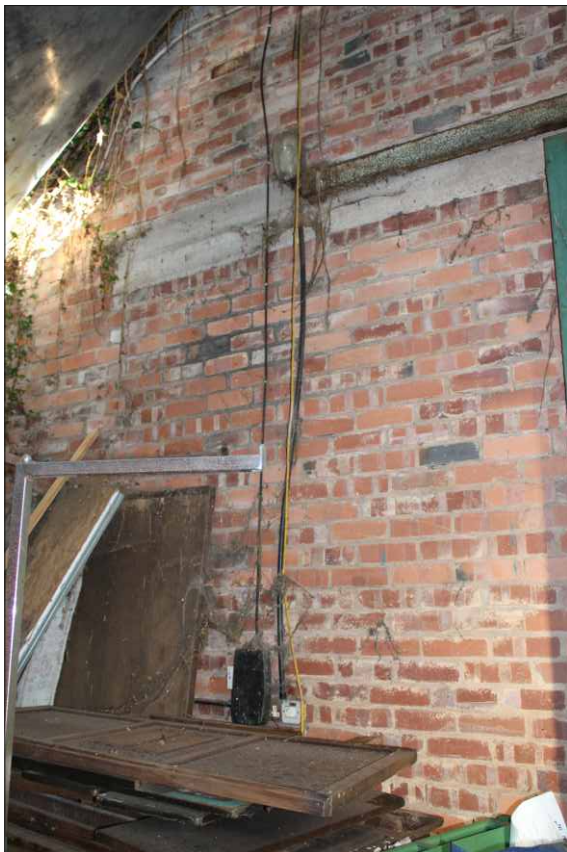
Plate 14: View of electrical fittings on the north wall of the Romney hut, looking northwest
