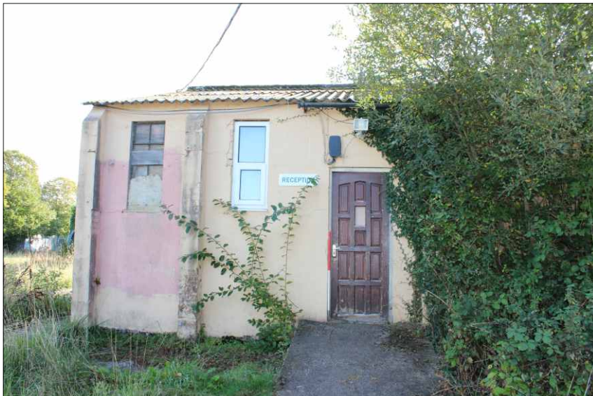
Plate 5: North end of the west elevation of the institute and NAAFI, looking east (1m scale)
