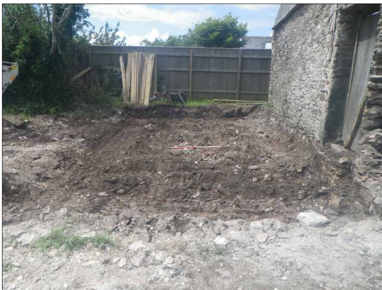
Plate 12: Area of watching brief in the area of the former western range, looking northwest (1m scale)
