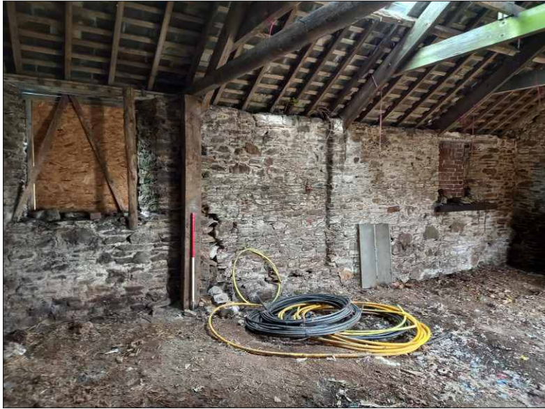
Plate 4: Internal view of north wall, showing blocked openings, looking north (1m scale)
