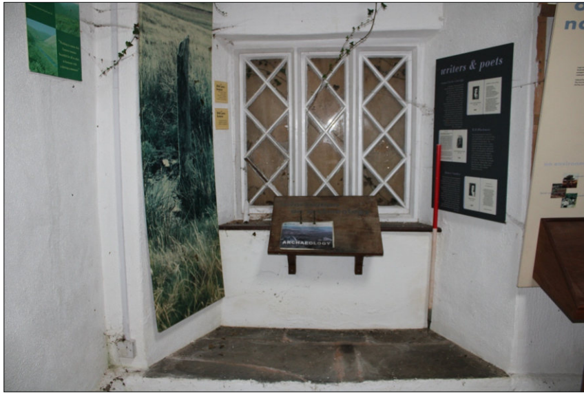
Plate 7: Internal view of north window in east elevation, looking southeast (1m scale)
