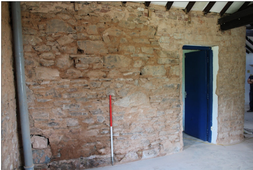
Plate 17: North wall of south extension, showing inserted doorway to right, looking northeast (1m scale)
