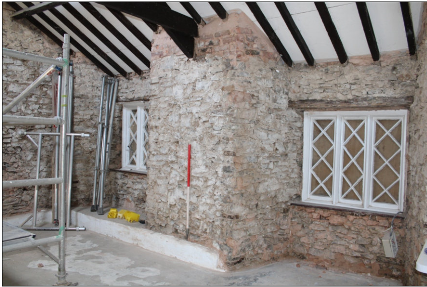
Plate 13: East wall with repointing visible particularly below the central window (on the right), looking east (1m scale)
