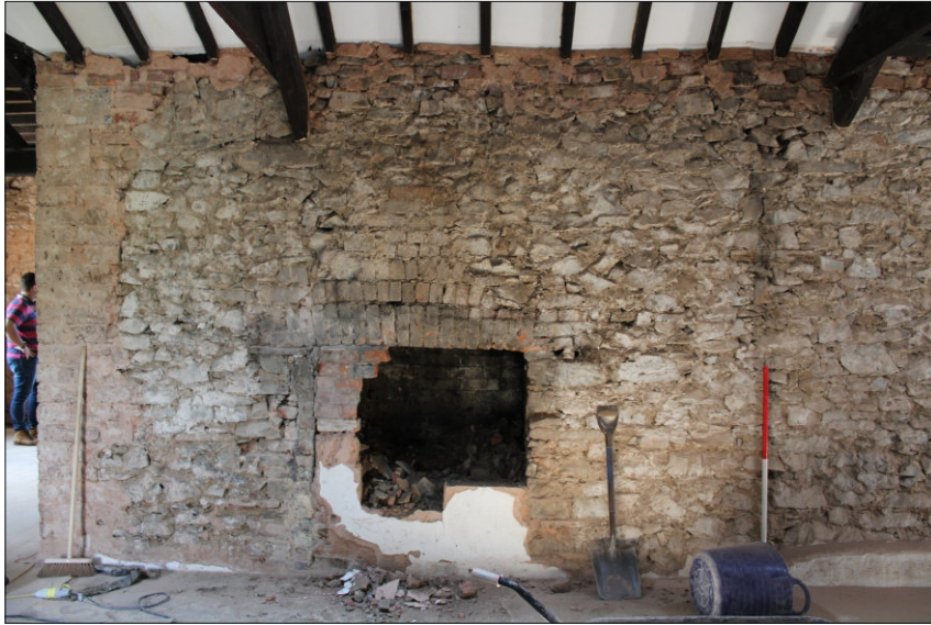
Plate 10: West wall showing wall scar to right, unblocked fireplace, centre and rebuilt wall to left, looking northwest (1m scale)
