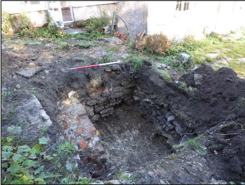
Plate 1: Oblique view of excavated trial pit. View from the south-west (scale 1m)
