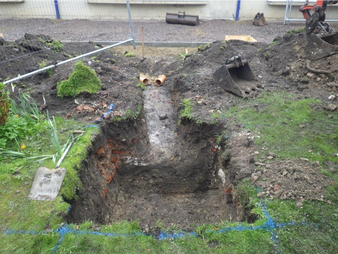
Plate 4:View of excavated soakaway (and trench) showing mortared bricks beneath the topsoil
