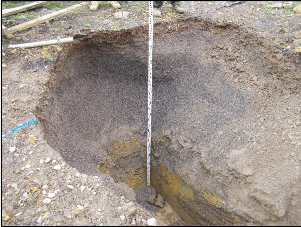
Plate 9: Depth of overburden material and instability of trench sides
