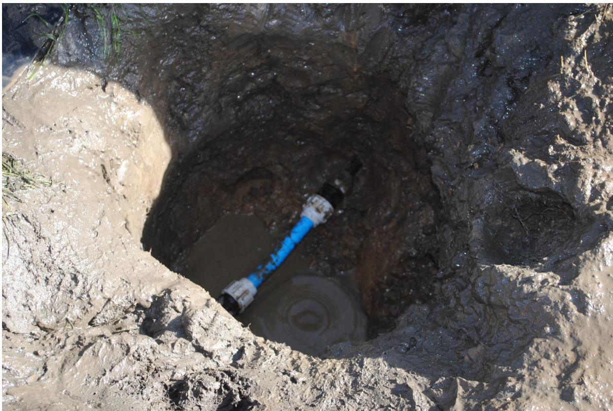
Plate 4: detail of completed pipe repair and full extents of access pit immediately prior to backfilling. View from south west
