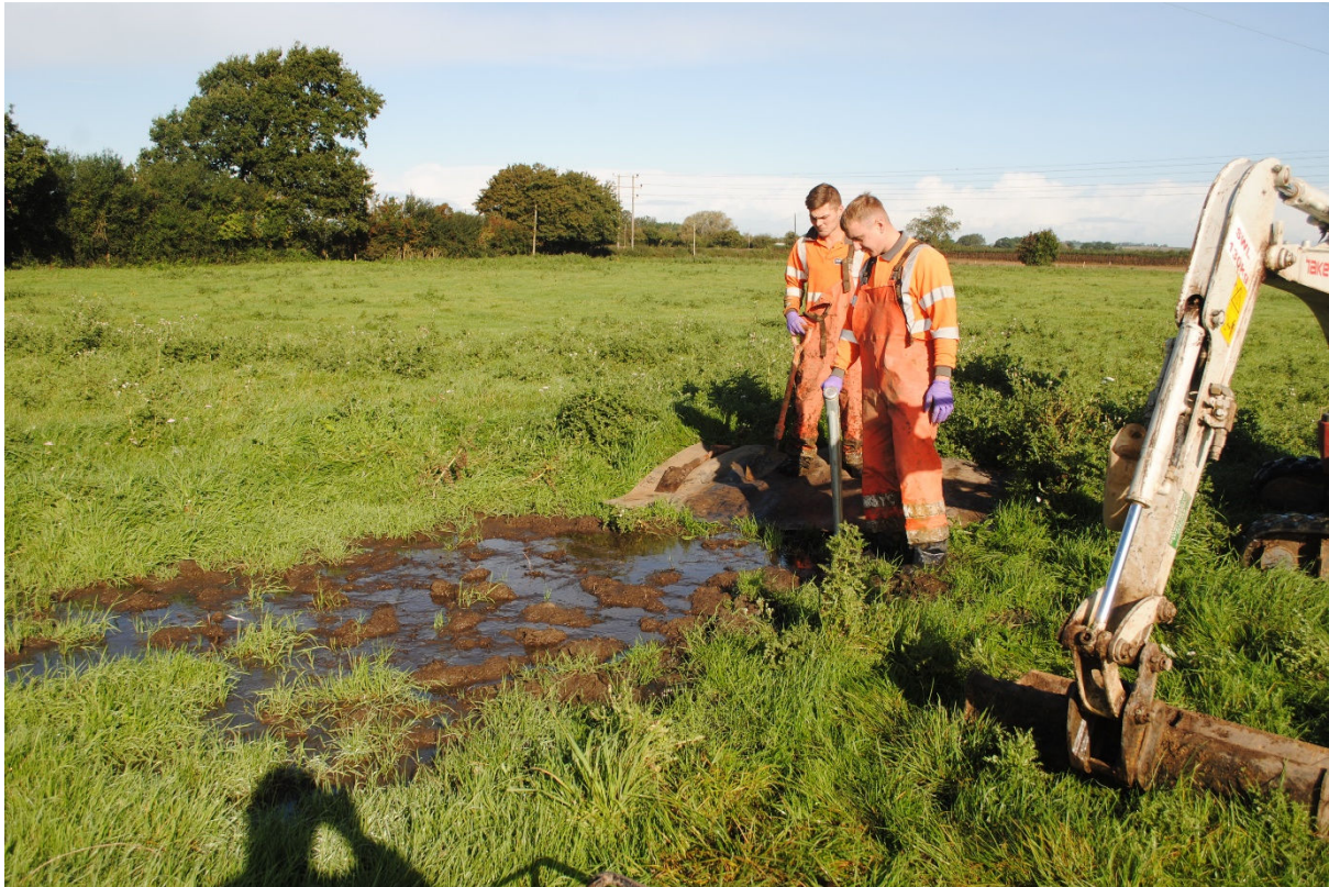
Plate 1: Condition of leak site on arrival. View from SSE
