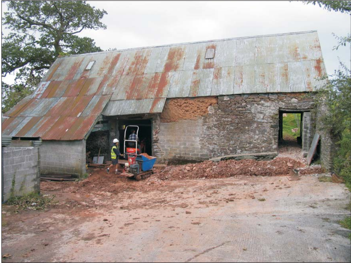
Plate 1: Eastern elevation of the building during early phases of groundworks. View to west
