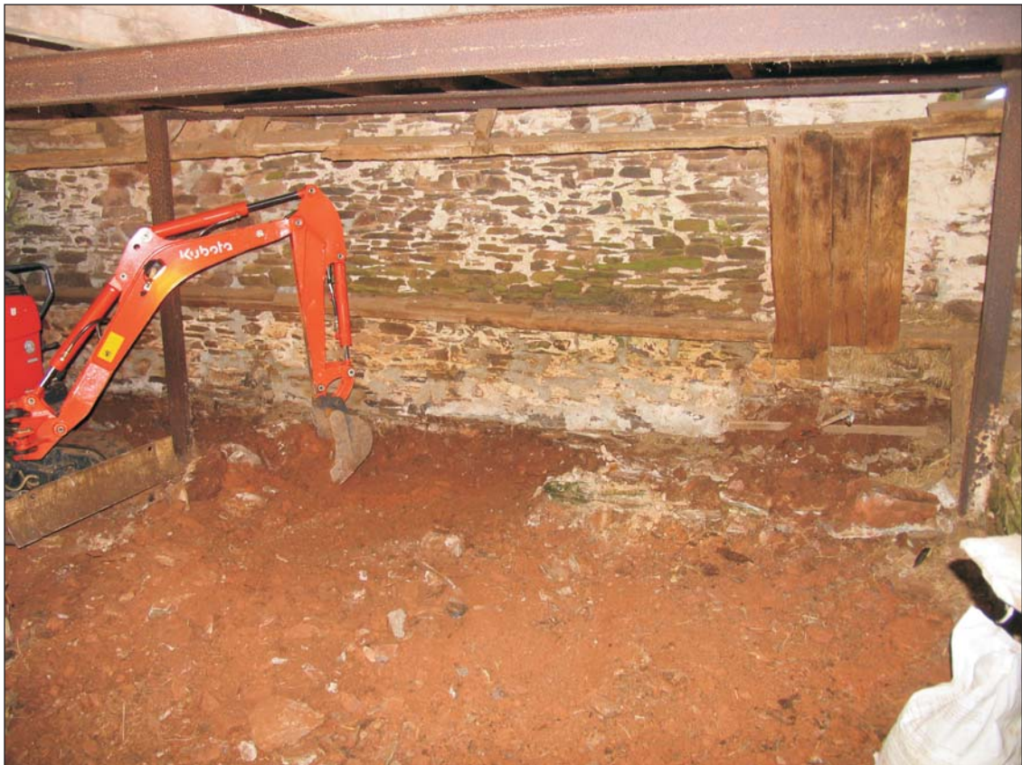
Plate 2: Interior of Lower Compartment following removal of cobbled floor. View to west
