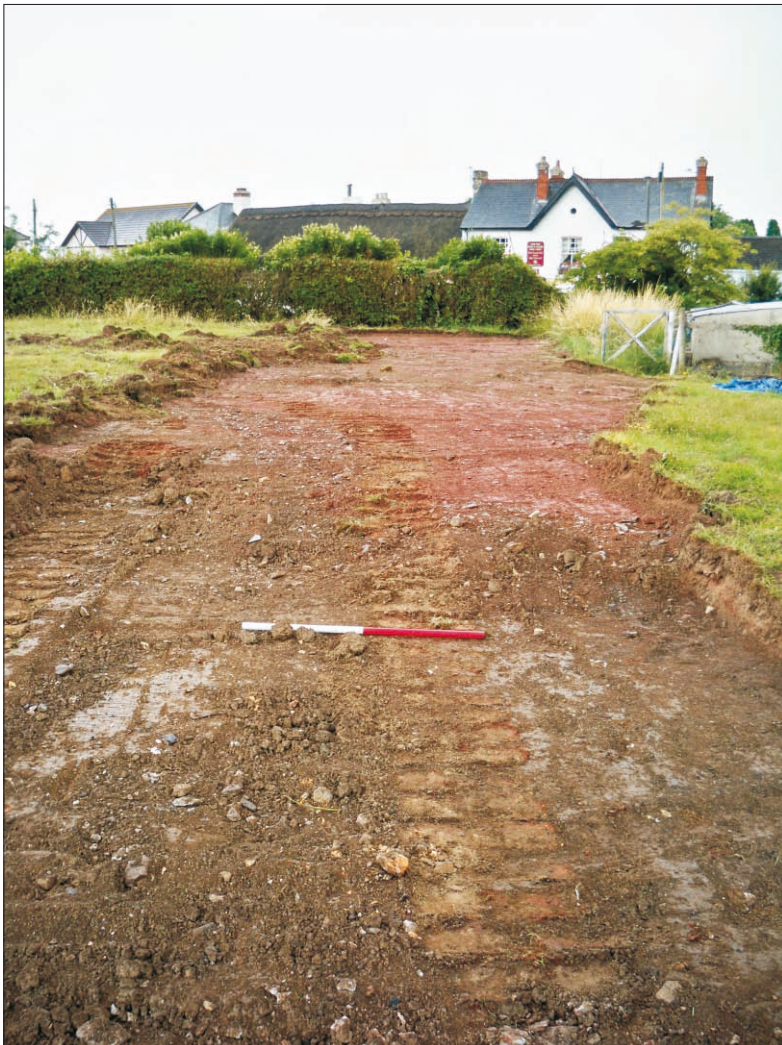
Plate 2: General view of site following partial soil strip, looking southwest (scale 1m)
