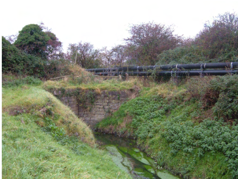
Plate 3. Drain crossed by railway line and overground pipelines at 3529018190. View to west
