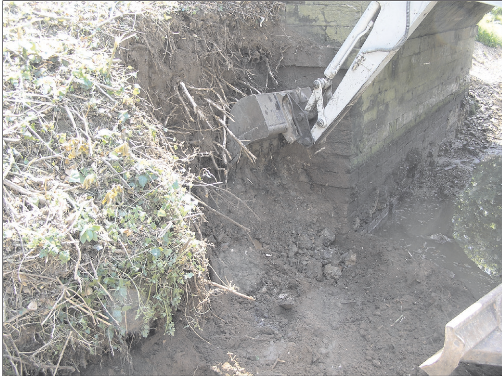
Plate 3: The removal of part of the east bank for sheet piling, view to southeast
