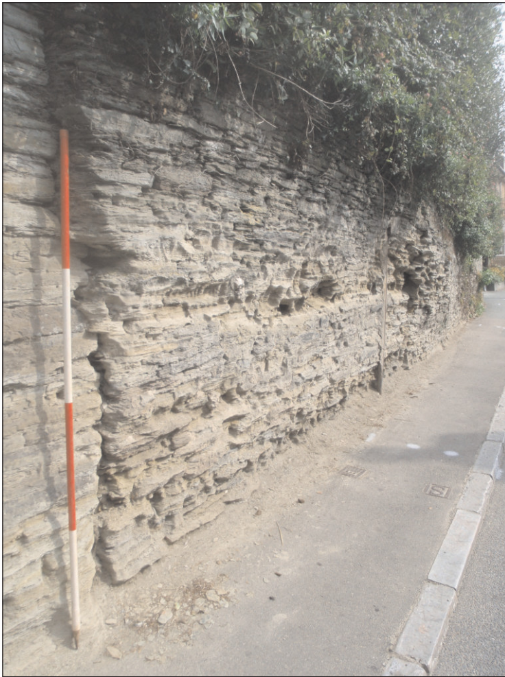
Plate 1: Detail of section of wall prior to its removal, view to northeast (Scale 2m).
