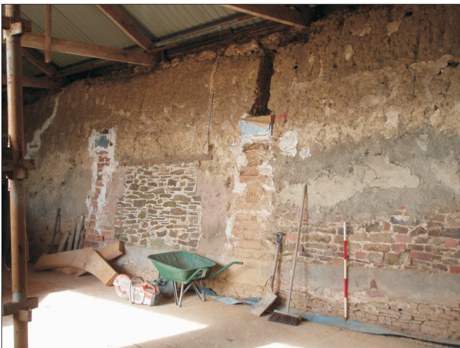
Plate 3. Internal view of the west wall of the barn, showing exposed stone and cob construction, brick and stone repairs and a blocked entrance. (Scale 1m)
