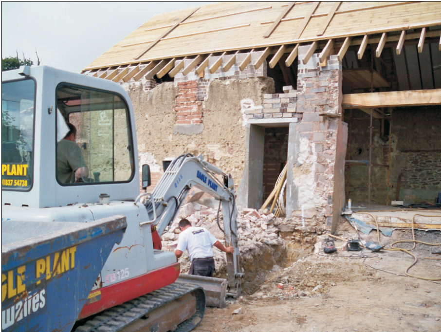
Plate 5. Excavation of the foundation trench to the southeast corner of the barn, view to the west.
