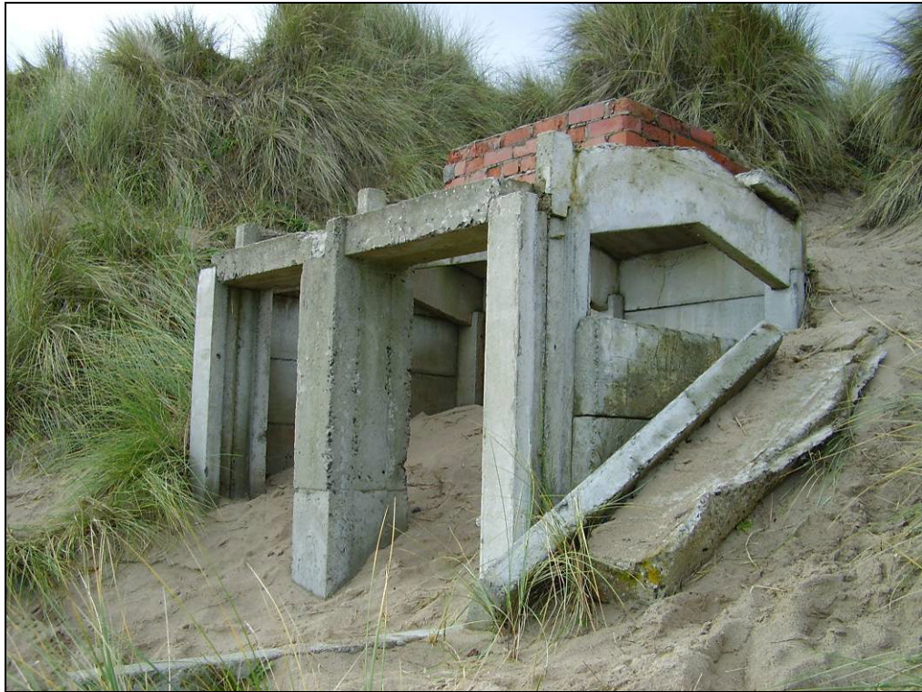
Fig 5.8.16 eroding military structure.
