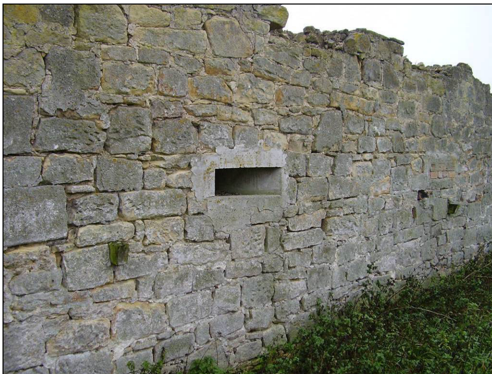
Fig 5.10.14 A Second World War loop hole placed in the wall of the post-medieval guano shed.
