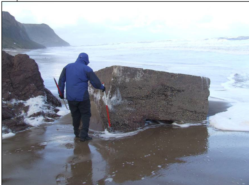
Figure 5.3.16 The same slumped pillbox as above more exposed to wave action, this time looking north. This photograph was taken in early December 2009 and demonstrates the changeable nature of the beach deposits and environmental conditions.
