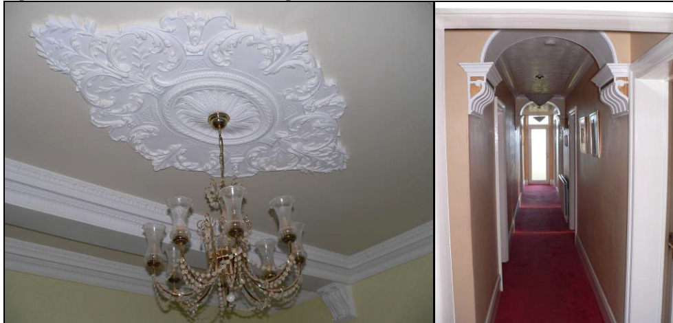
Fig 5.7.9 Internal features including the chandelier, indicating the higher status of the Officer's Mess and a view of the corbelling in the main corridor.
