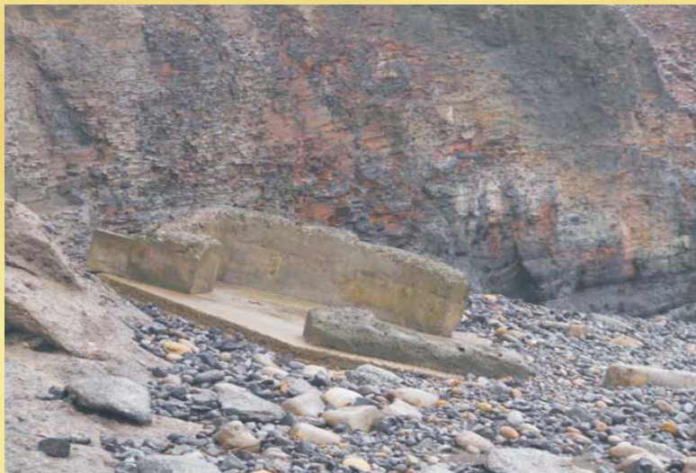
The remains of a Second World War pillbox, destroyed due to coastal erosion of the cliffs at Sandsend, North Yorkshire
