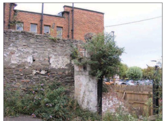
f) Standing remains in Area 3, looking southeast, illustrating the sudden drop to Unity Street.
