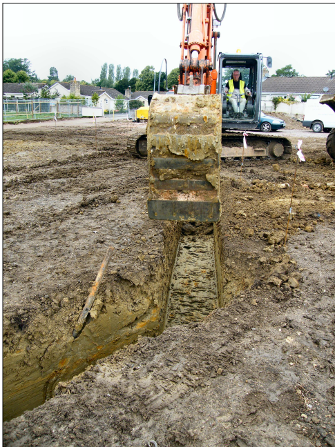
C) Detail of the car park boundary wall during excavation. Viewed from the southeast.
