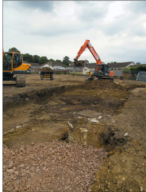
B) Southern end of the access road during excavation, Manhole 4 in the foreground Cut 116 in the background. Viewed from the southwest.
