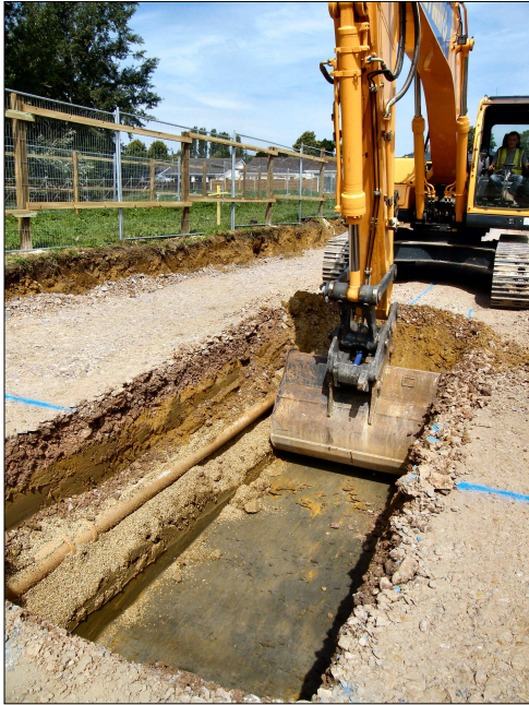
A) Detail of the access road during the excavation of the replacement foul water pipe, showing the undisturbed natural substrate. Viewed from the south.
