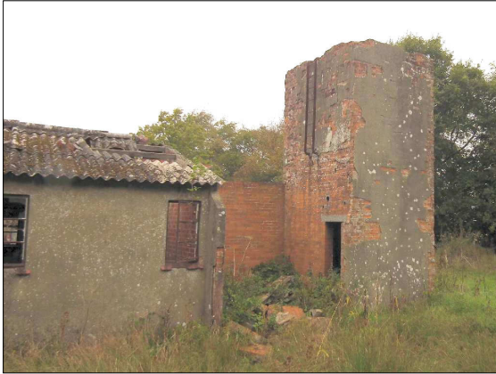
Plate a. The north end of Structure 1 with the tower attached, looking northwest.
