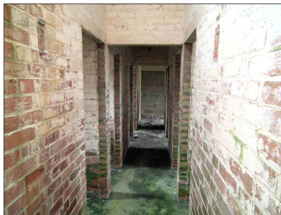
Plate d. Interior of Structure 1, looking north, showing central corridor with cubicles on either side.
